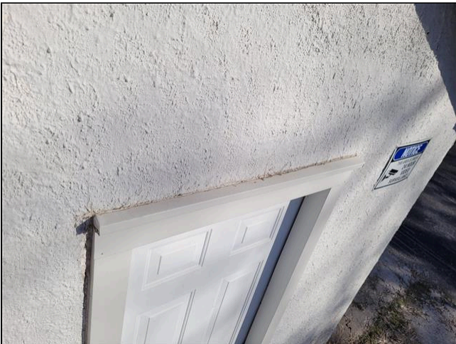
2.1 Item 11(Picture) No Z flashing-doors
