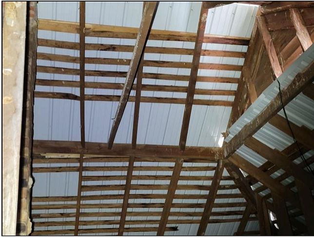
4.4 Item 3(Picture) Missing purlins
