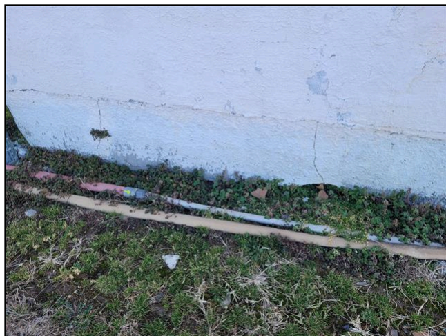
4.0 Item 3(Picture) Cracks
