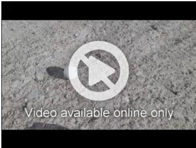
2.5 Item 3(Video) Improper grading
