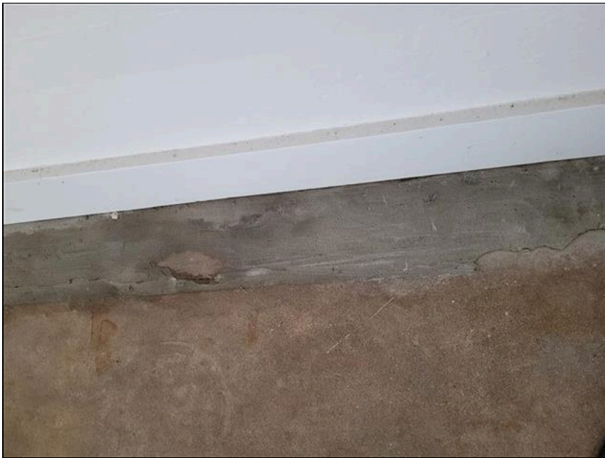
4.0 Item 5(Picture) Exterior wall-slab area not continuous
