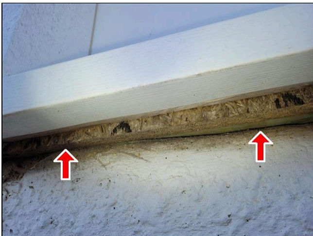
2.1 Item 9(Picture) No visible flashing
