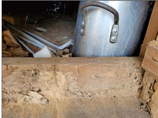
3.7 Item 4(Picture) Wood destroying insect activity
