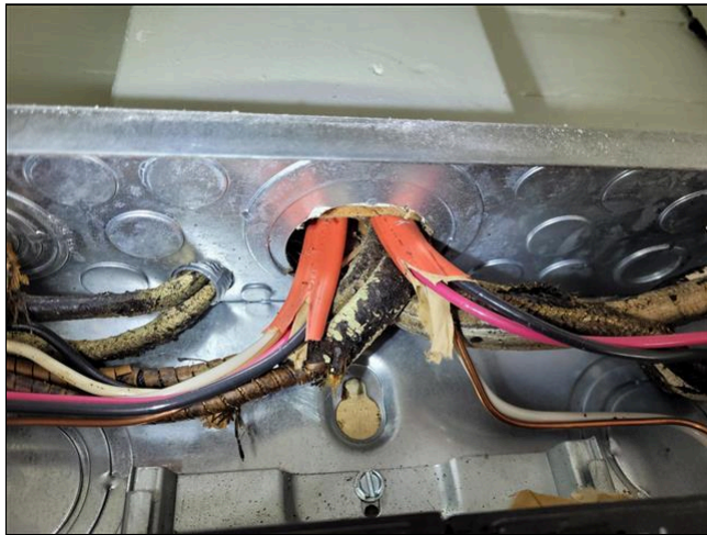
6.1 Item 3(Picture) Bushing needed
