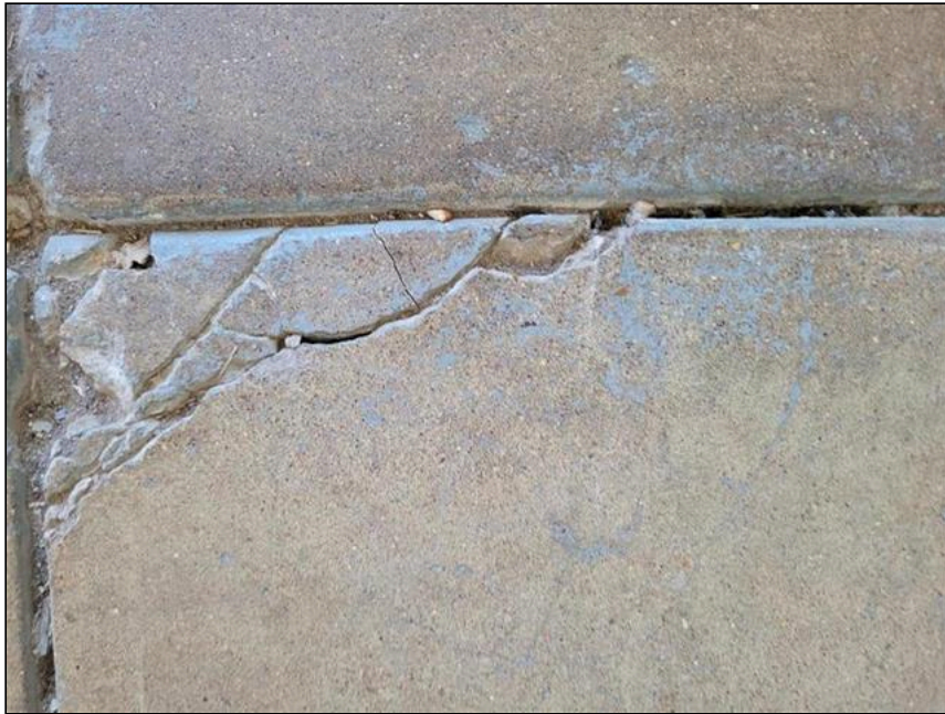
3.2 Item 6(Picture) Floor-damage
