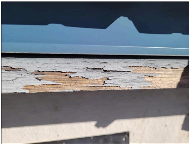
2.0 Item 7(Picture) Scrape/paint-as needed
