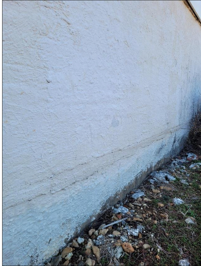
2.0 Item 2(Picture) Possible bulging
