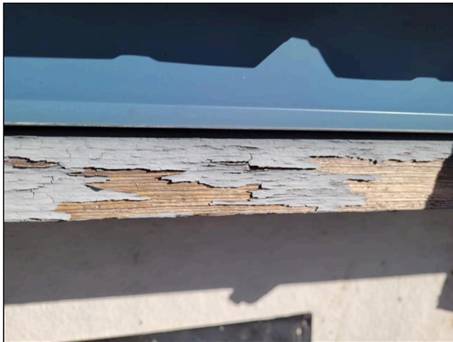
2.0 Item 7(Picture) Scrape/paint-as needed
