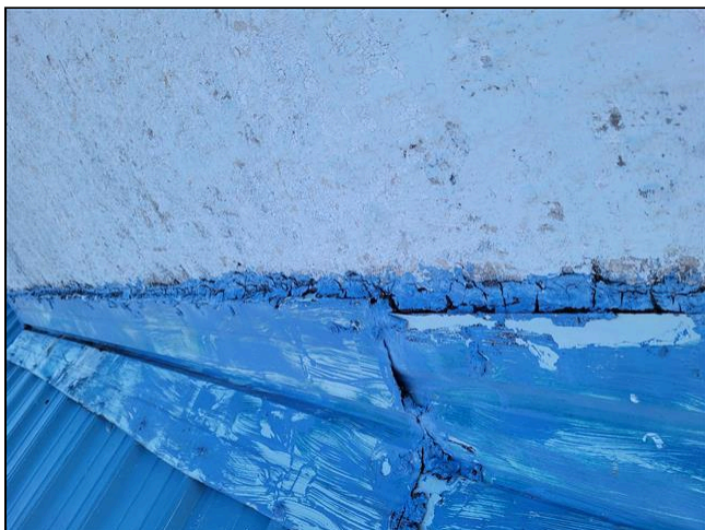
1.1 Item 7(Picture) Cracked sealant
