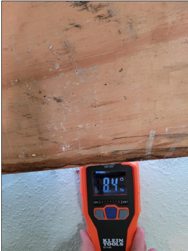
3.6 Item 3(Picture) East school room window area-low moisture reading
