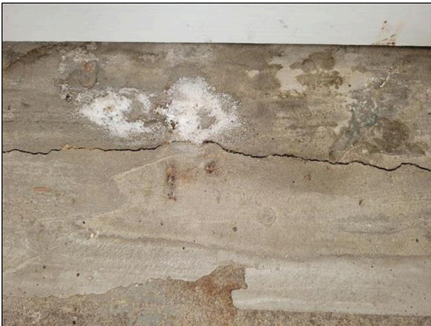
3.2 Item 4(Picture) Floor-settling cracks
