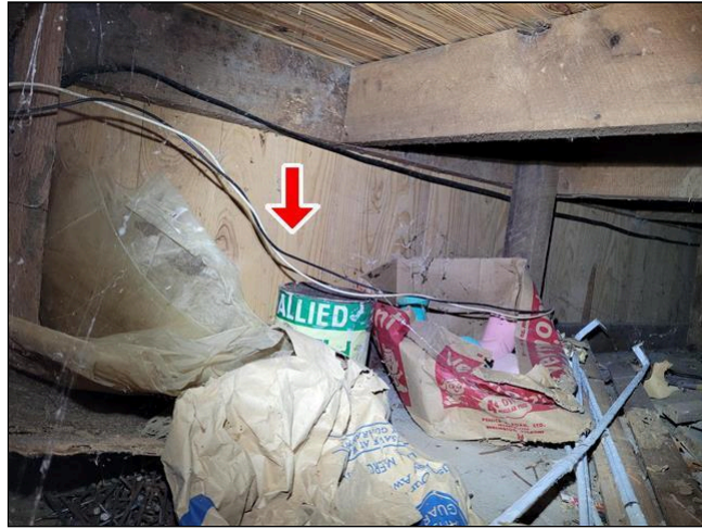
6.2 Item 4(Picture) Exposed wiring-conduit needed
