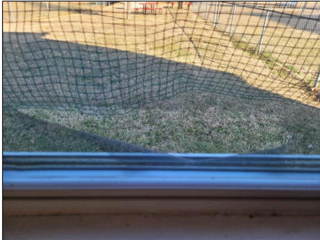
3.6 Item 1(Picture) Window exterior screens-damaged
