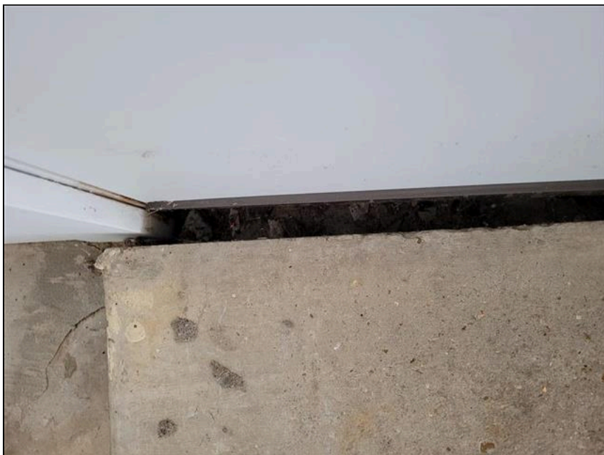
3.2 Item 5(Picture) Entry door floor-gap
