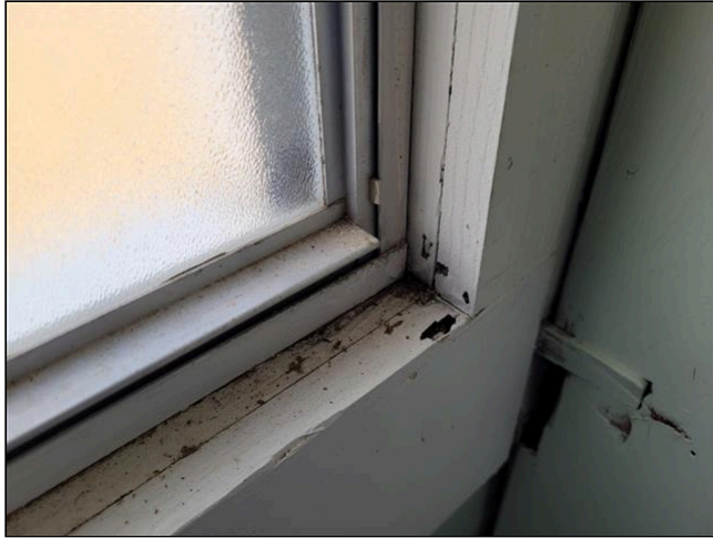
3.4 Item 1(Picture) Damaged window trim-bathroom
