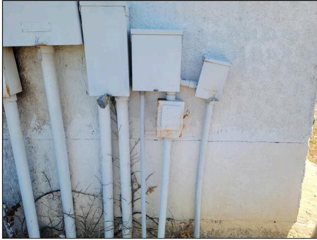
2.0 Item 1(Picture) Cracked exterior
