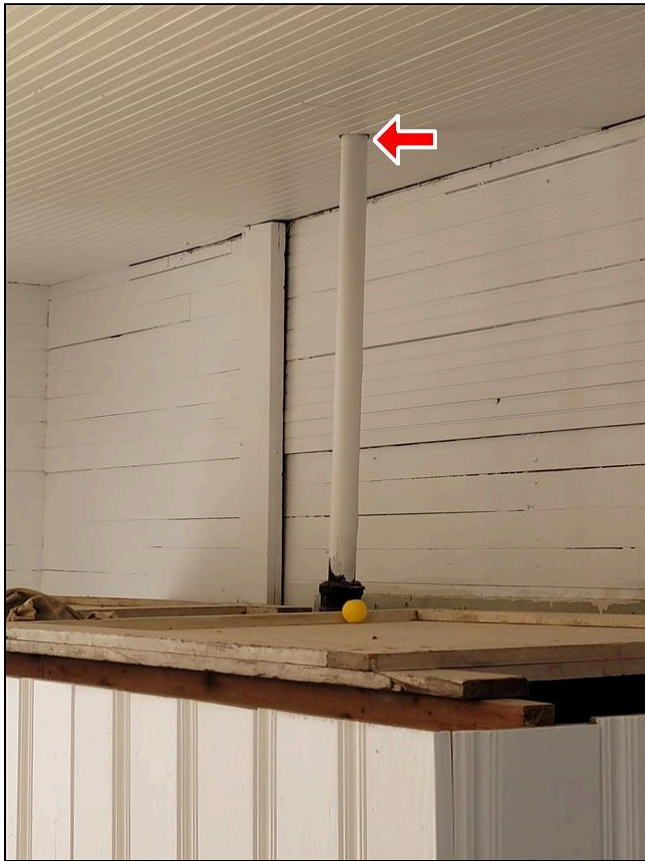
5.0 Item 1(Picture) DWV pipe-not exiting roof area
