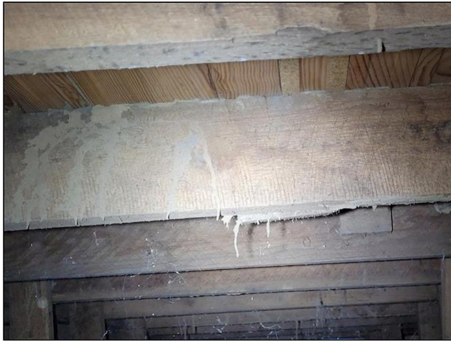
3.7 Item 1(Picture) Wood destroying insect activity
