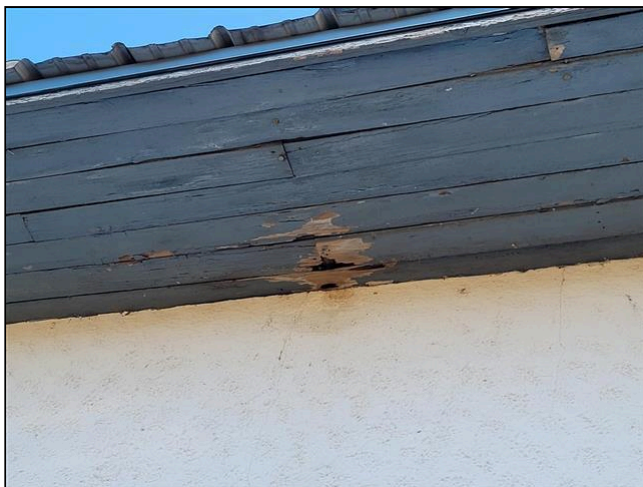
2.4 Item 5(Picture) Damaged soffit material
