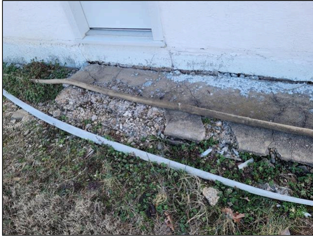
2.5 Item 4(Picture) Damaged concrete
