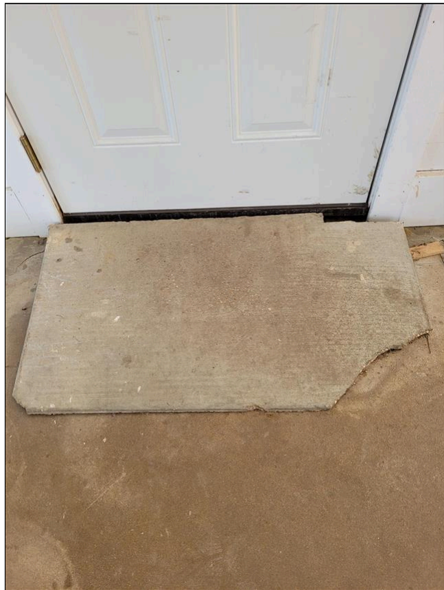
3.2 Item 9(Picture) Front door ramp-loose
