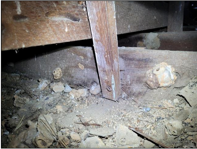
4.4 Item 7(Picture) Improper roof support anchoring method
