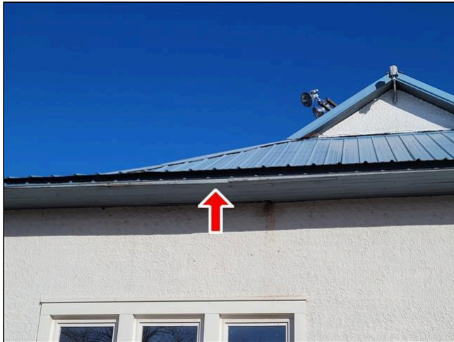
2.4 Item 3(Picture) Dropping fascia
