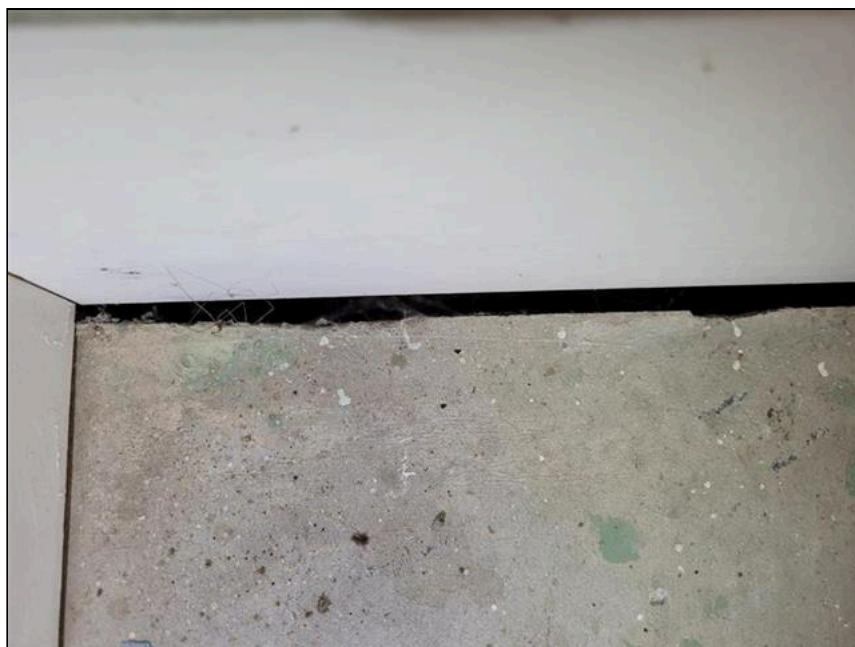
3.2 Item 3(Picture) Floor-gap in concrete
