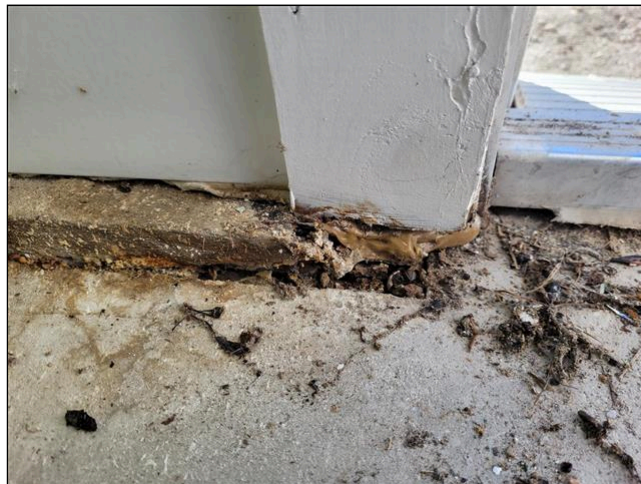
4.0 Item 2(Picture) Wood destroying insect activity
