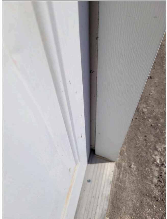
2.1 Item 8(Picture) Unsealed door-Southeast door
