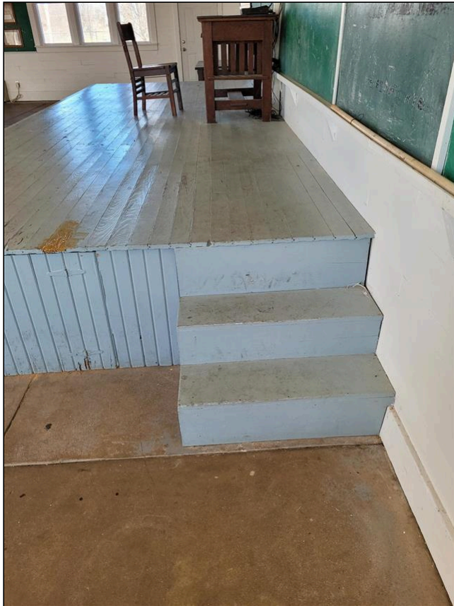
3.3 Item 1(Picture) Handrail-needed for the stage
