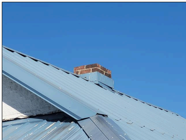
7.4 Item 1(Picture) No visible chimney cap
