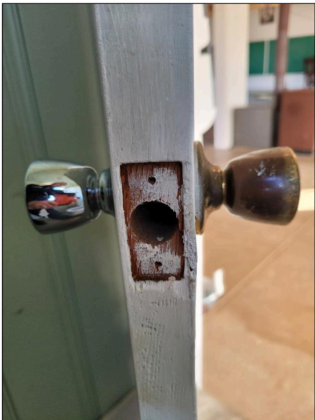
3.5 Item 3(Picture) Women's bathroom door-missing latch
