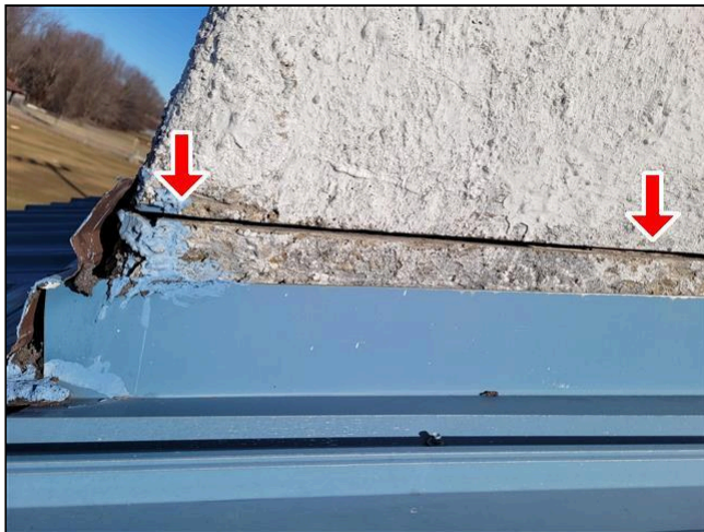
1.1 Item 5(Picture) Flash/seal all areas properly/ missing flashing
