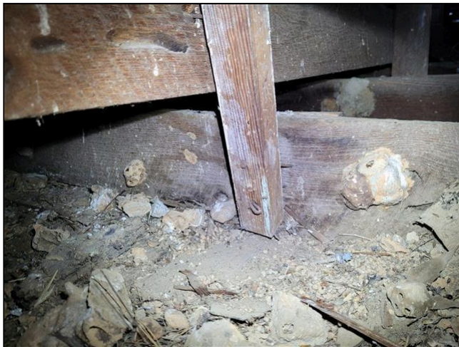
4.4 Item 7(Picture) Improper roof support anchoring method
