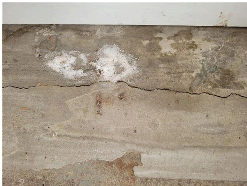
3.2 Item 4(Picture) Floor-settling cracks
