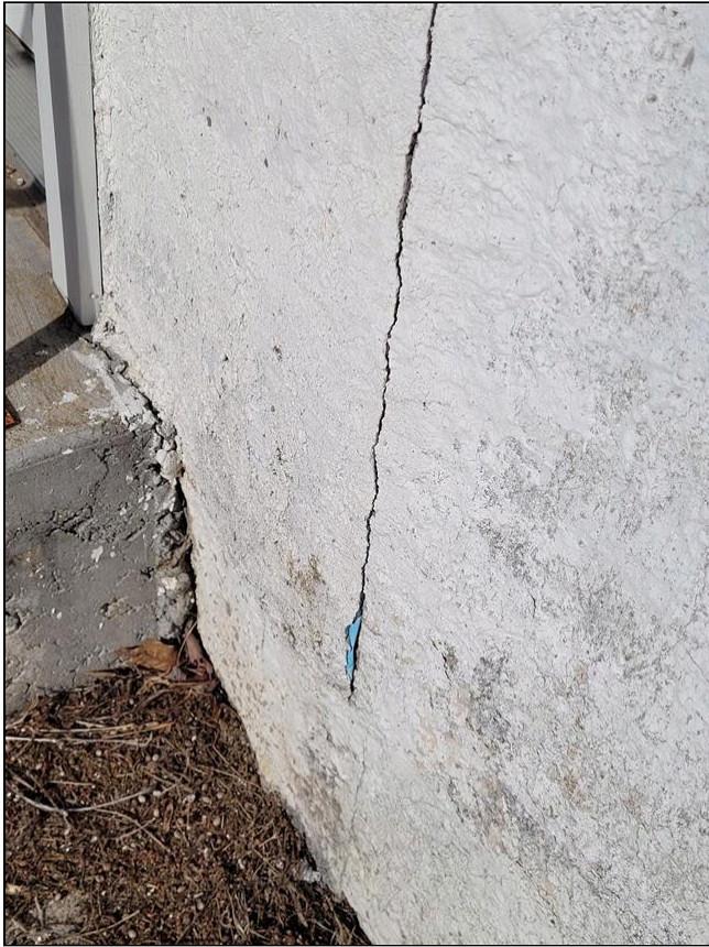
2.0 Item 5(Picture) Cracked exterior
