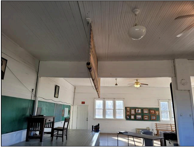
3.0 Item 3(Picture) Main beam-appears to be sagging
