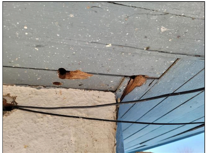
2.4 Item 2(Picture) Aged soffit material
