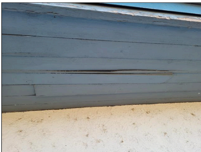
2.4 Item 7(Picture) Aged soffit material
