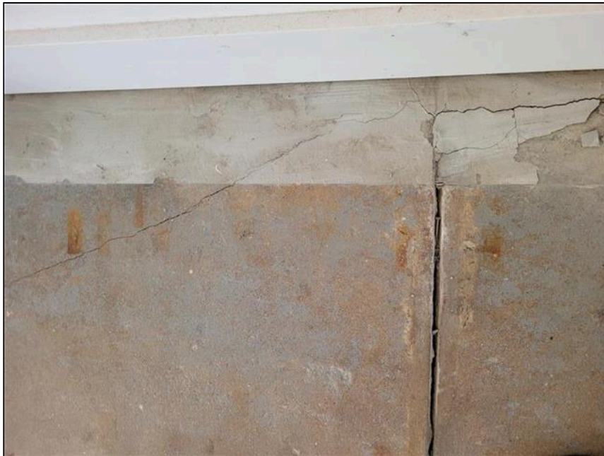
3.2 Item 7(Picture) Floor-settling cracks
