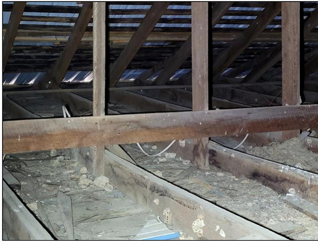
4.4 Item 5(Picture) Improper framing method
