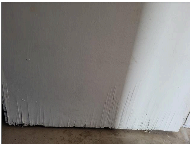
3.5 Item 4(Picture) Women's bathroom door-damaged
