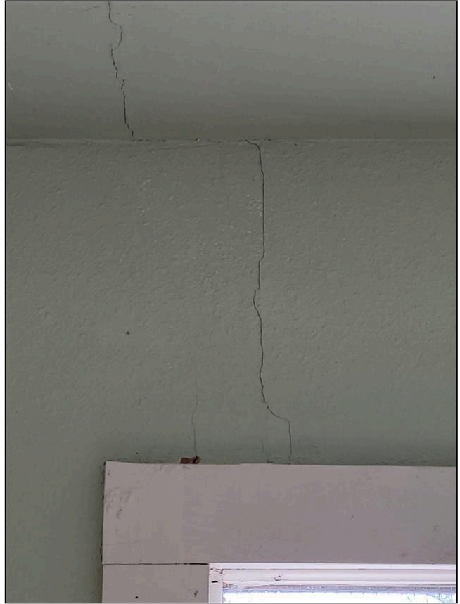
3.1 Item 2(Picture) East school room wall-settling cracks
