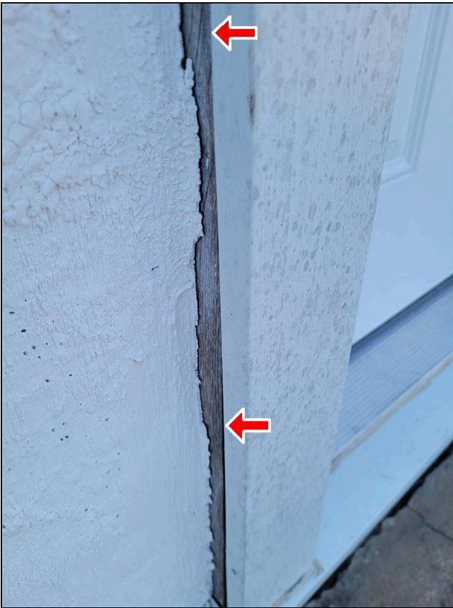
2.1 Item 10(Picture) Exposed wood
