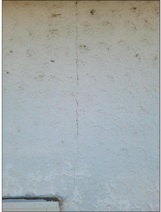
2.0 Item 6(Picture) Cracked exterior
