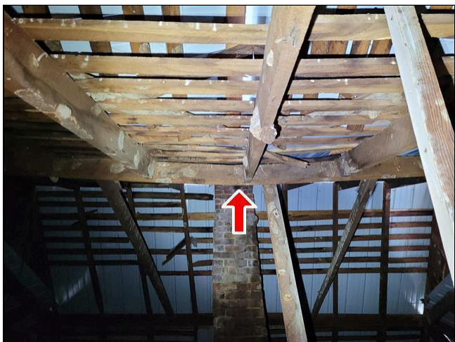
4.4 Item 1(Picture) Sagging framing area/incorrect anchoring method
