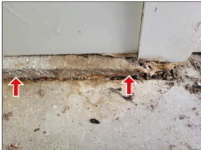
4.0 Item 1(Picture) Wood-no visible concrete footing
