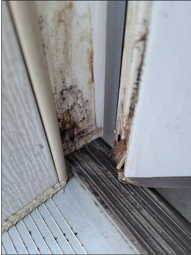
2.1 Item 5(Picture) Rotten jamb, rotten door-North door
