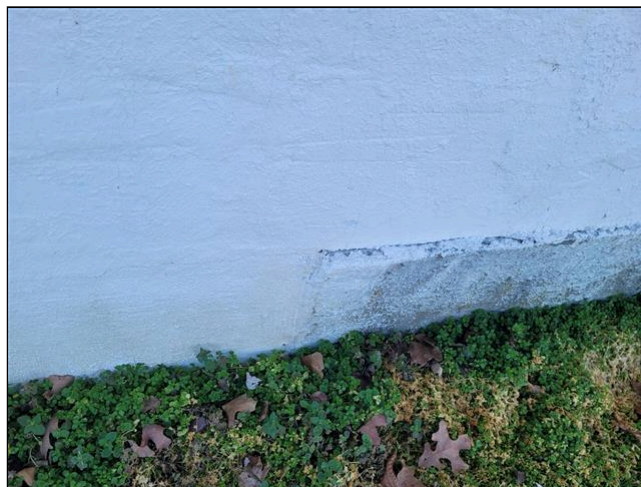
4.0 Item 4(Picture) Cracks
