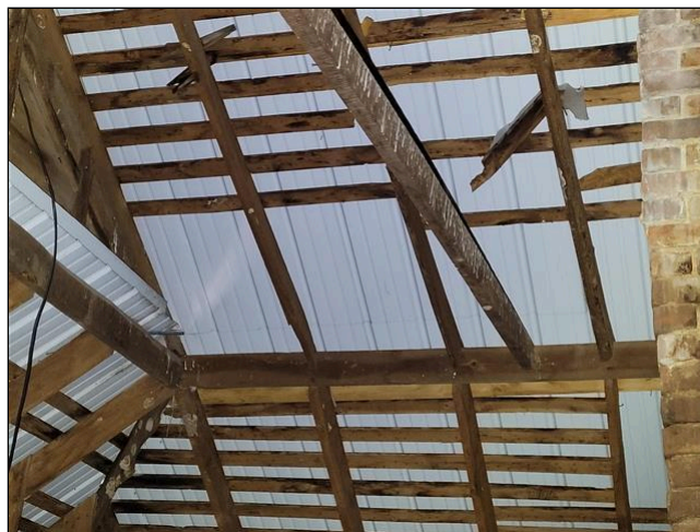
4.4 Item 2(Picture) Missing purlins
