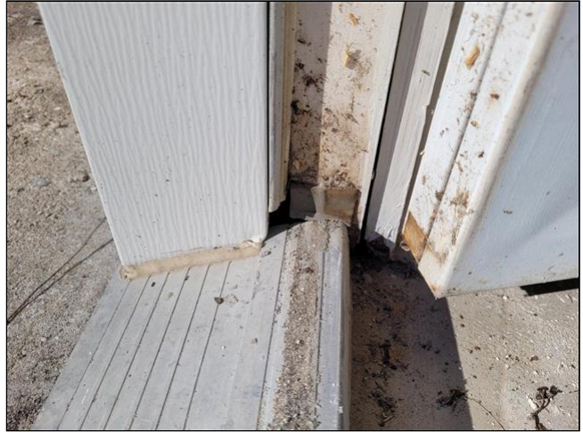
2.1 Item 2(Picture) Rotten jamb-Southeast side
