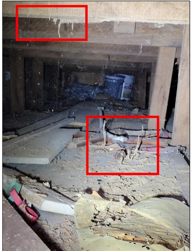
3.7 Item 2(Picture) Wood destroying insect activity
