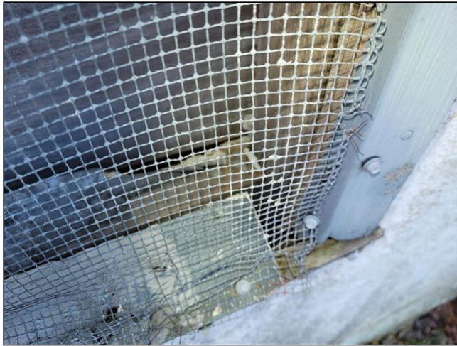
2.2 Item 3(Picture) Missing pane-North side
