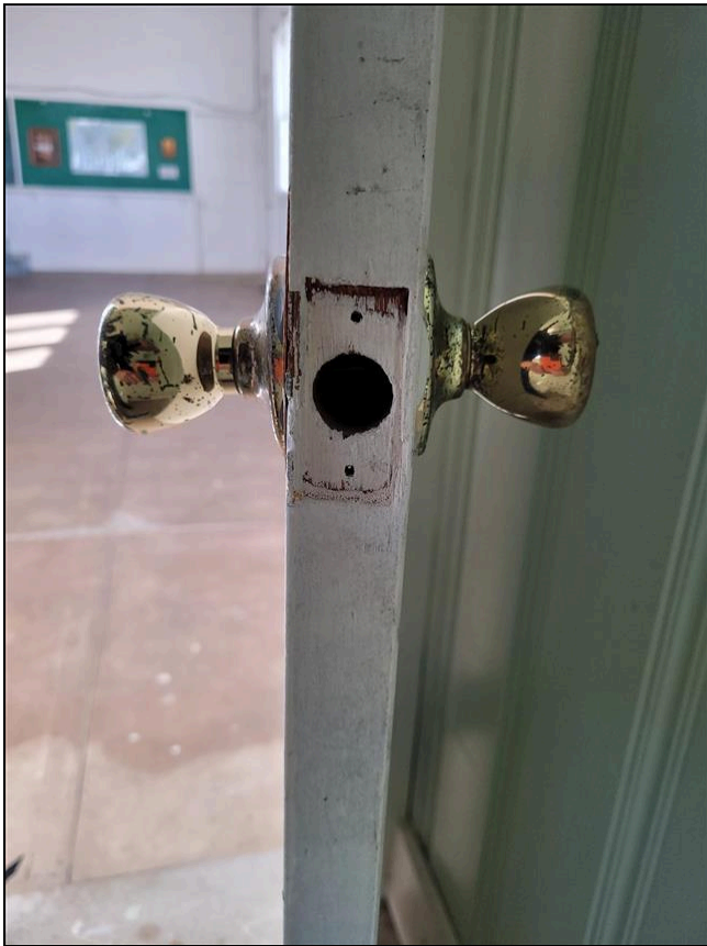
3.5 Item 1(Picture) Men's bathroom door-missing latch
