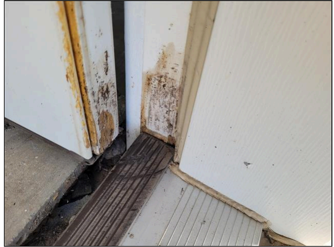
2.1 Item 6(Picture) Water intrusion-South door
