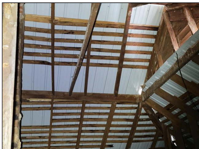
4.4 Item 3(Picture) Missing purlins
