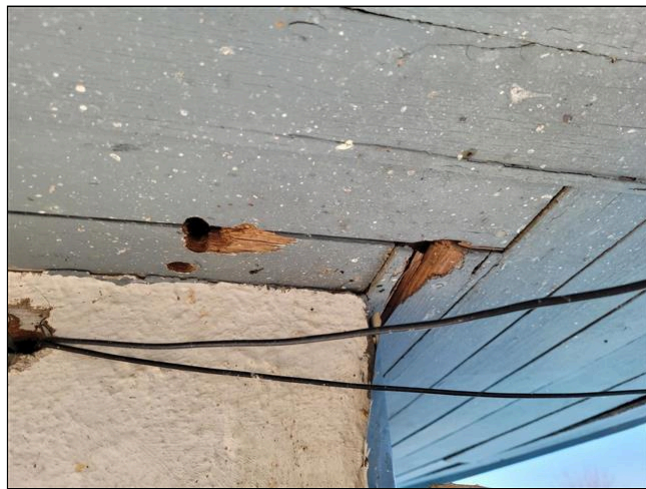
2.4 Item 2(Picture) Aged soffit material
