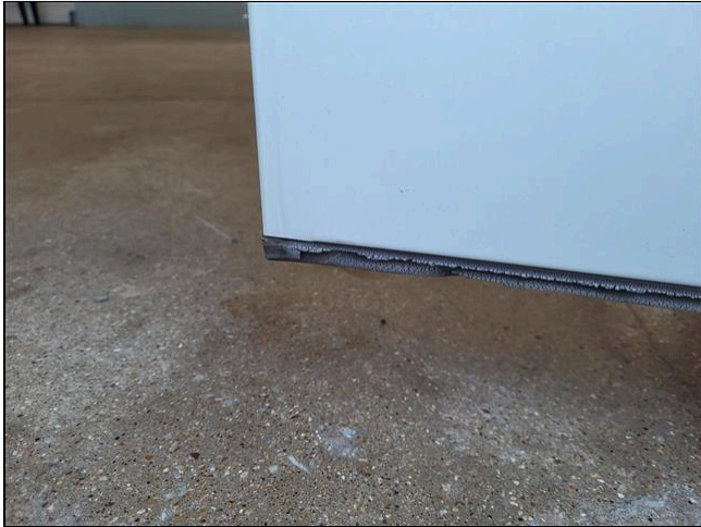
2.1 Item 7(Picture) Replace all damaged threshold seals
