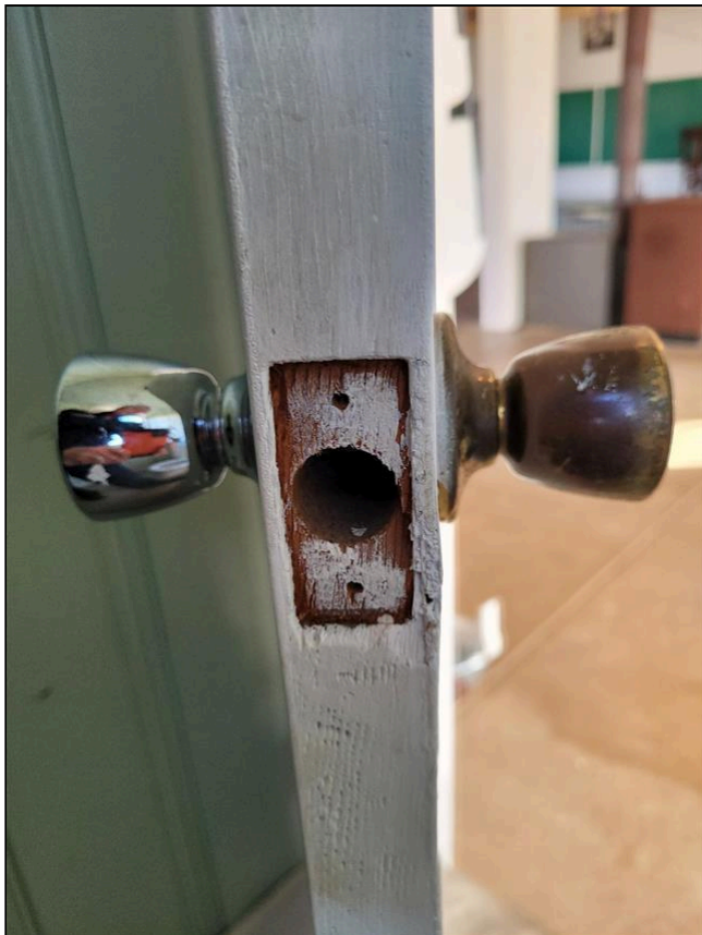
3.5 Item 3(Picture) Women's bathroom door-missing latch
