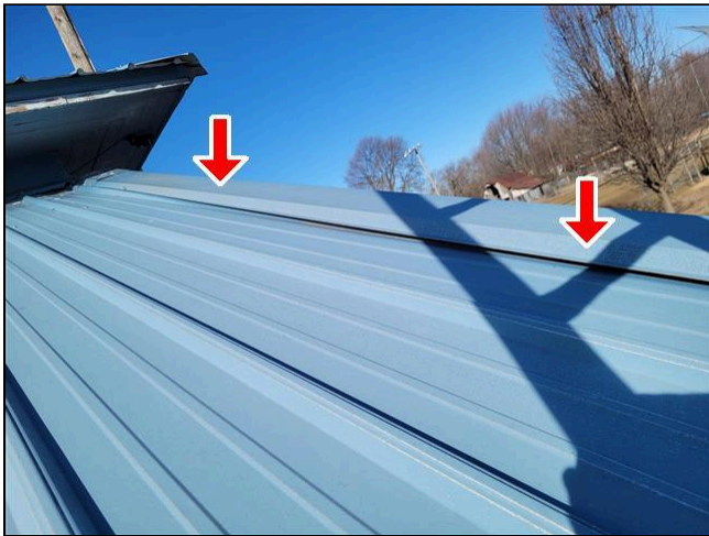
1.0 Item 4(Picture) Missing screws
