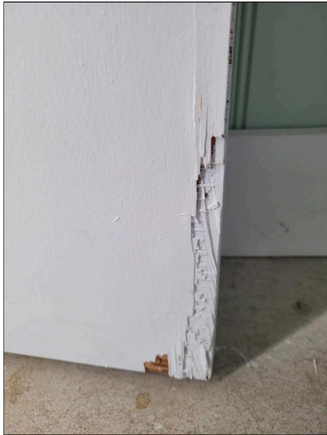
3.5 Item 2(Picture) Men's bathroom door-damaged
