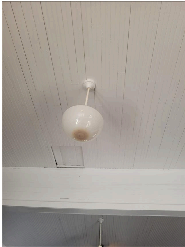
6.2 Item 2(Picture) Main area light-did not work
