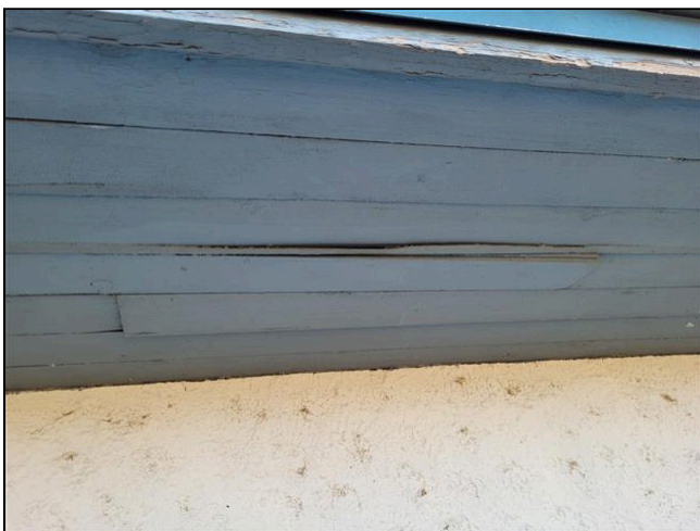
2.4 Item 7(Picture) Aged soffit material
