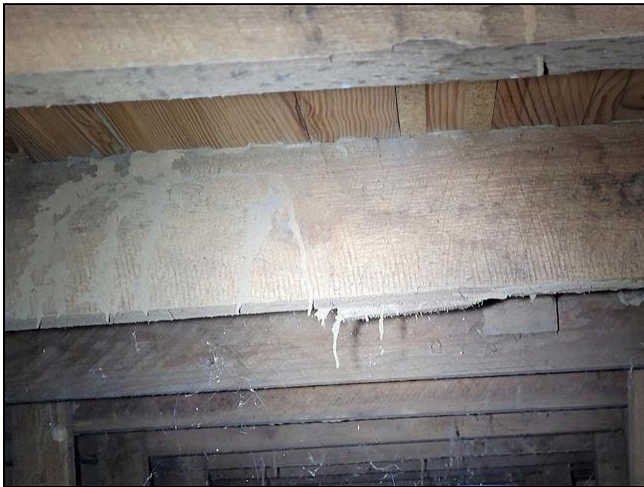
3.7 Item 1(Picture) Wood destroying insect activity
