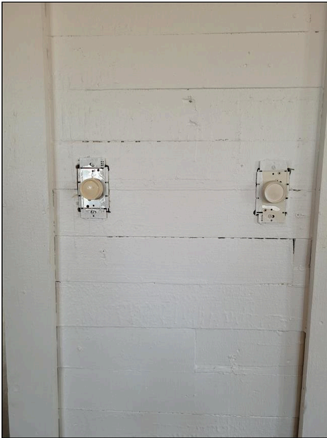
6.2 Item 1(Picture) Dimmer switches-overheating/no switch covers
