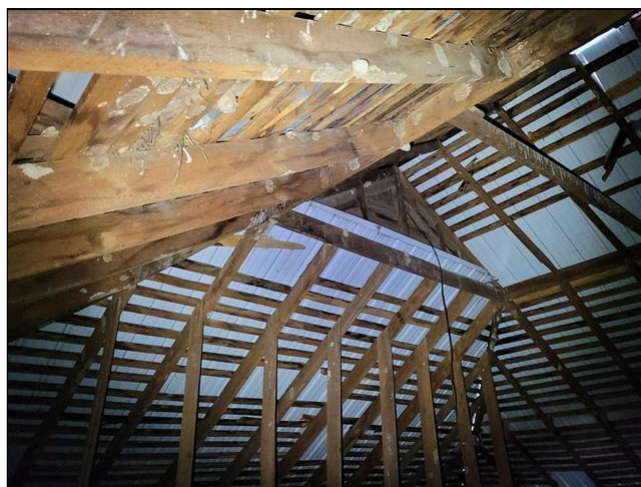
4.4 Item 4(Picture) Missing purlins
