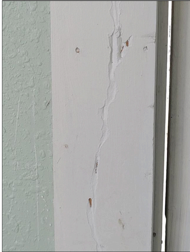
3.4 Item 2(Picture) East school room trim-possible would destroying insect damage
