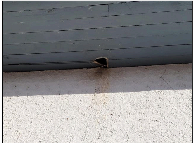
2.4 Item 4(Picture) Hole-soffit
