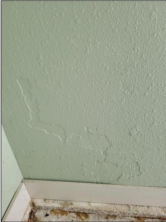
3.1 Item 3(Picture) East school room wall-possible wood destroying insect damage
