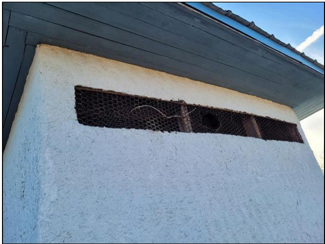
8.1 Item 1(Picture) Damaged attic vent material
