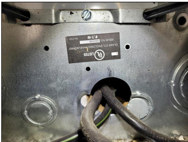
6.1 Item 4(Picture) Bushing needed
