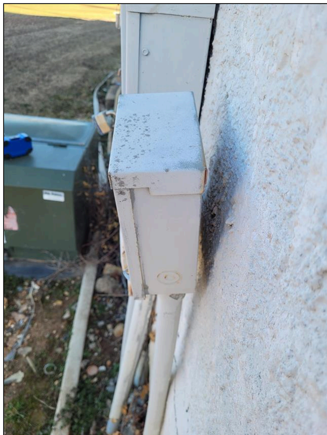
6.1 Item 8(Picture) Anchor disconnect panel
