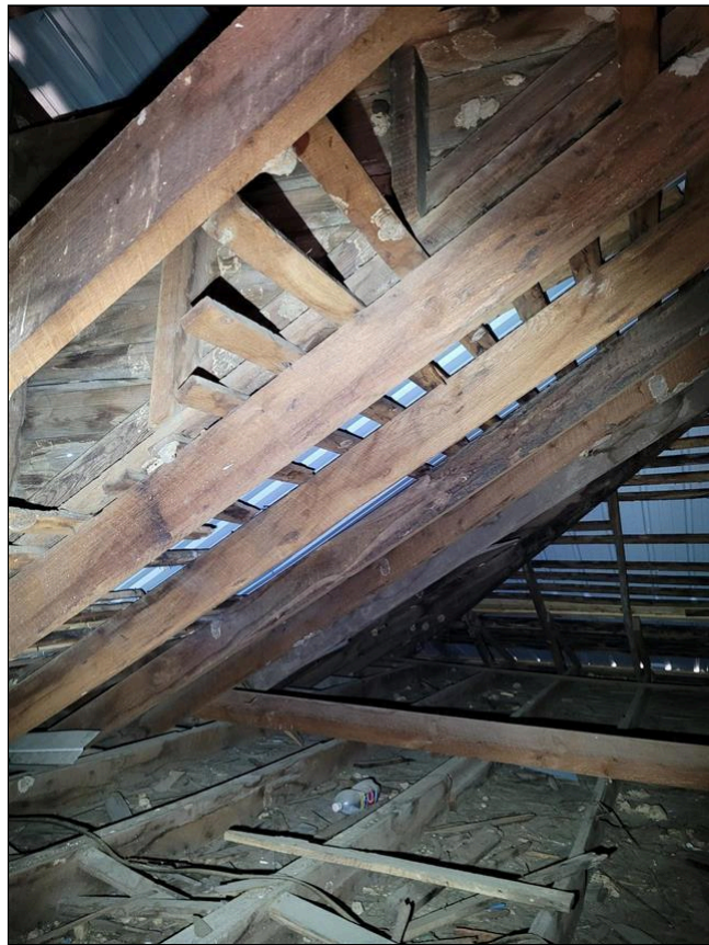
4.4 Item 6(Picture) Missing roof supports
