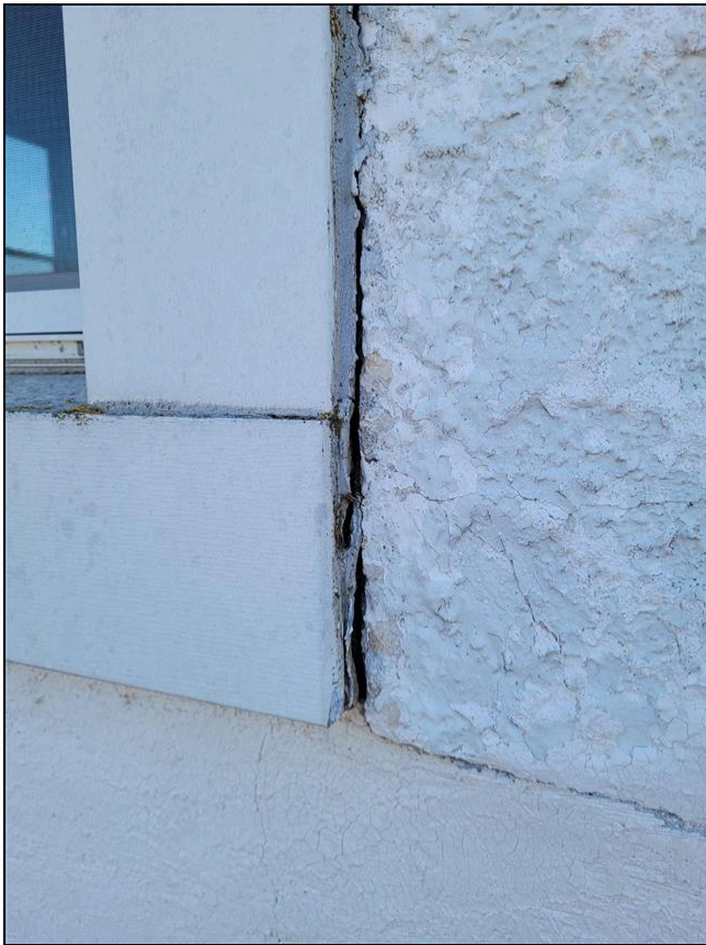
2.2 Item 1(Picture) Sealant needed-windows
