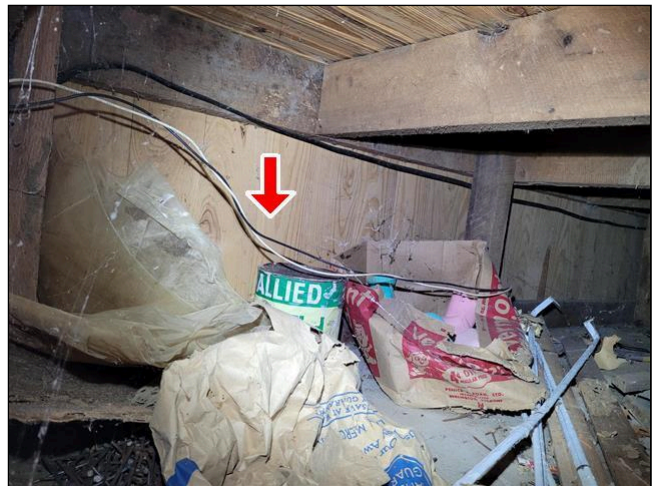
6.2 Item 4(Picture) Exposed wiring-conduit needed
