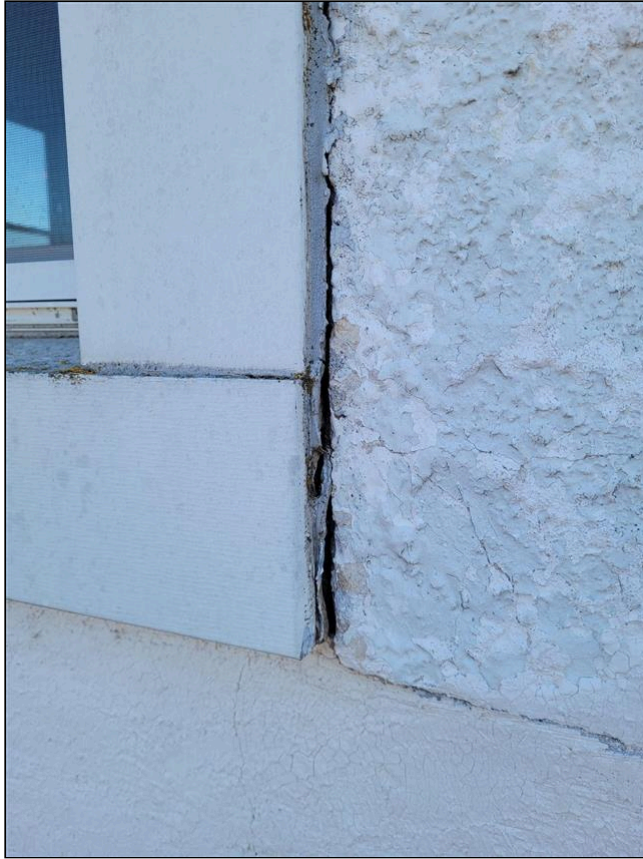
2.2 Item 1(Picture) Sealant needed-windows
