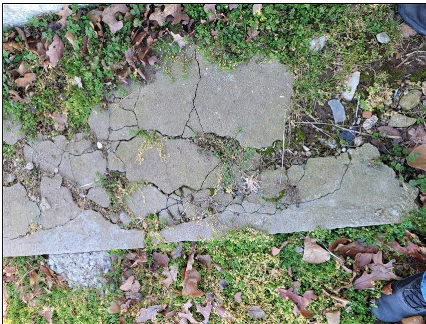
2.5 Item 5(Picture) Damaged concrete
