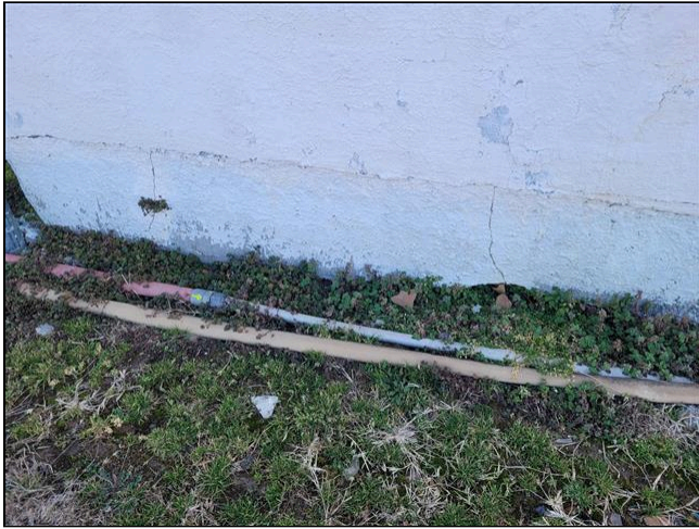
4.0 Item 3(Picture) Cracks
