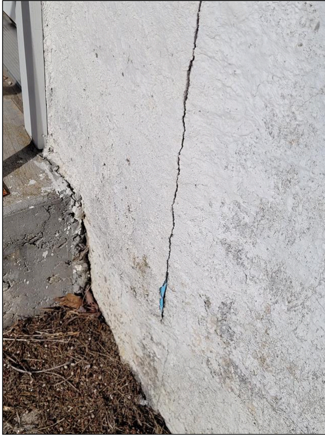
2.0 Item 5(Picture) Cracked exterior
