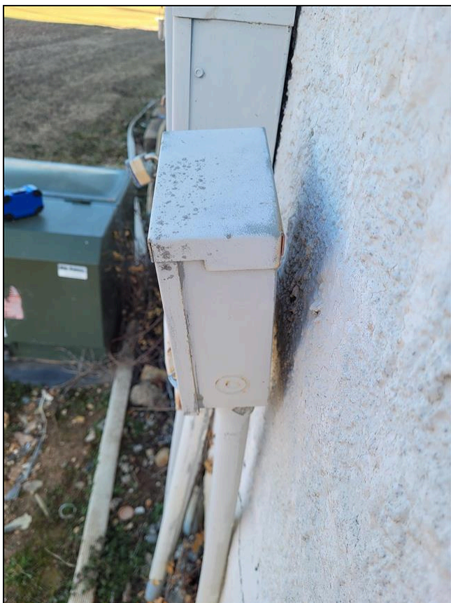
6.1 Item 8(Picture) Anchor disconnect panel
