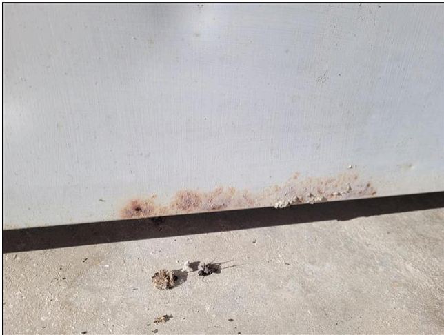
2.1 Item 3(Picture) Rust holes-Southeast side
