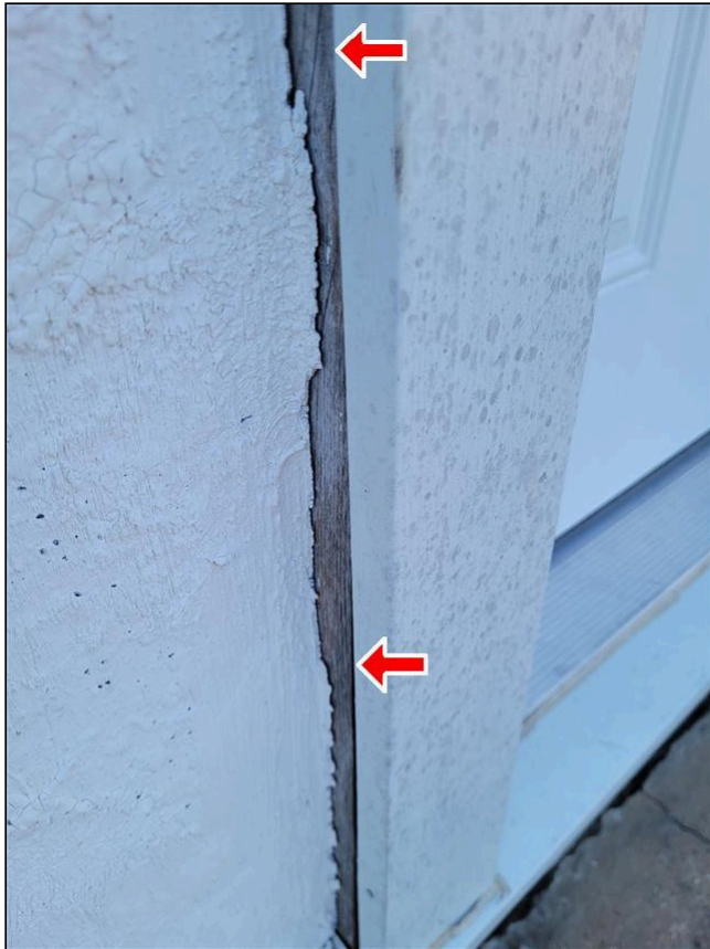
2.1 Item 10(Picture) Exposed wood
