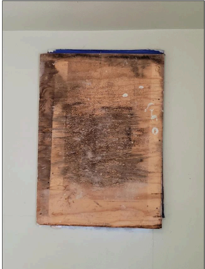
3.6 Item 2(Picture) East school room window-missing pane
