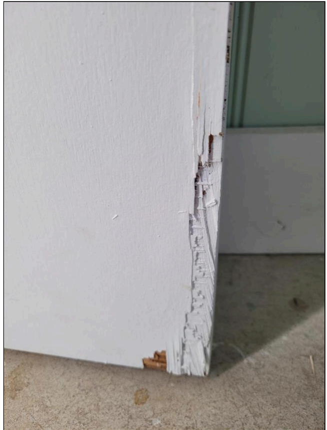
3.5 Item 2(Picture) Men's bathroom door-damaged
