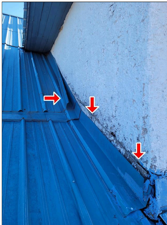
1.1 Item 8(Picture) Loose/missing flashing
