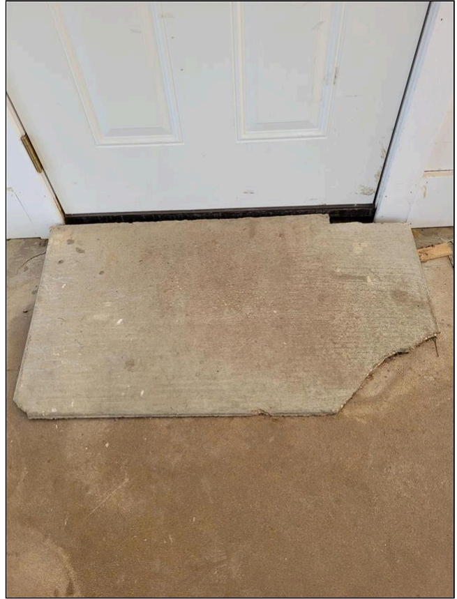
3.2 Item 9(Picture) Front door ramp-loose
