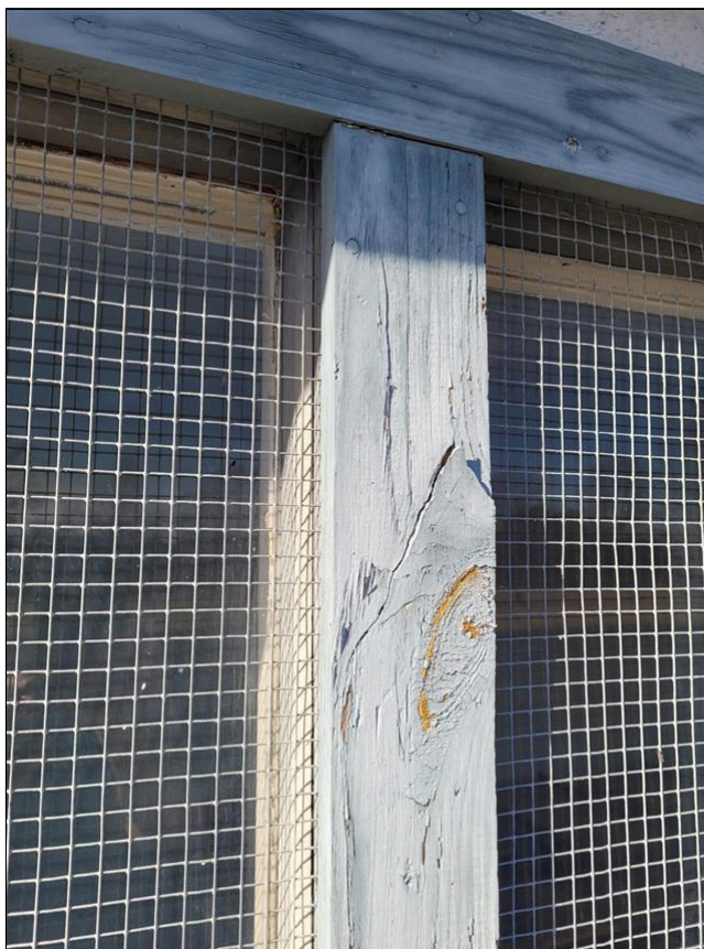
2.2 Item 6(Picture) Aged window trim
