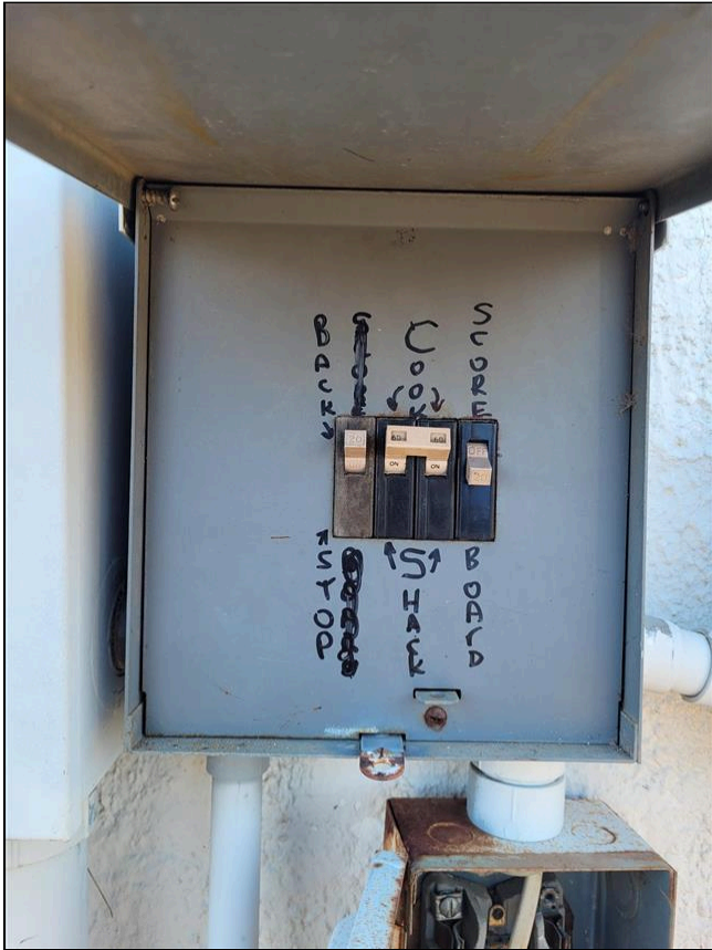
6.1 Item 7(Picture) Score board breaker-turned off, not tested
