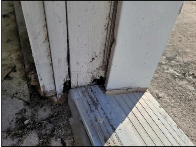
2.1 Item 1(Picture) Rotten jamb-Southeast side
