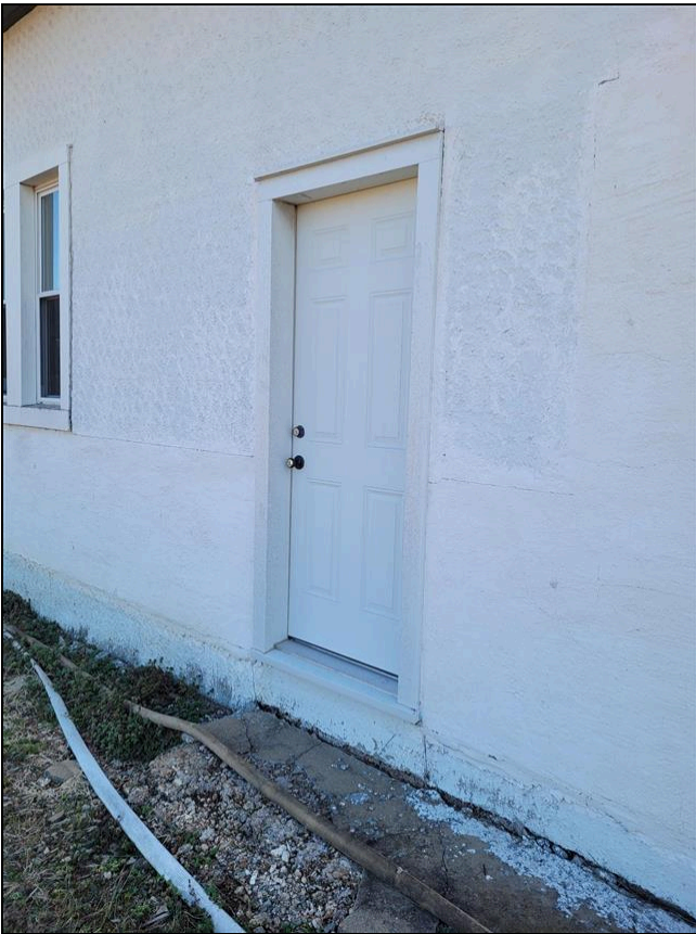
2.3 Item 1(Picture) Step and handrail needed-West side
