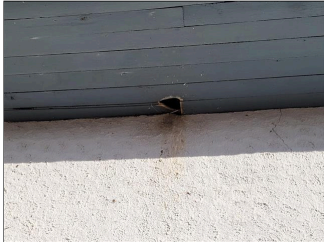
2.4 Item 4(Picture) Hole-soffit
