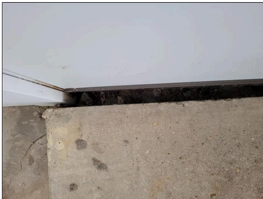
3.2 Item 5(Picture) Entry door floor-gap
