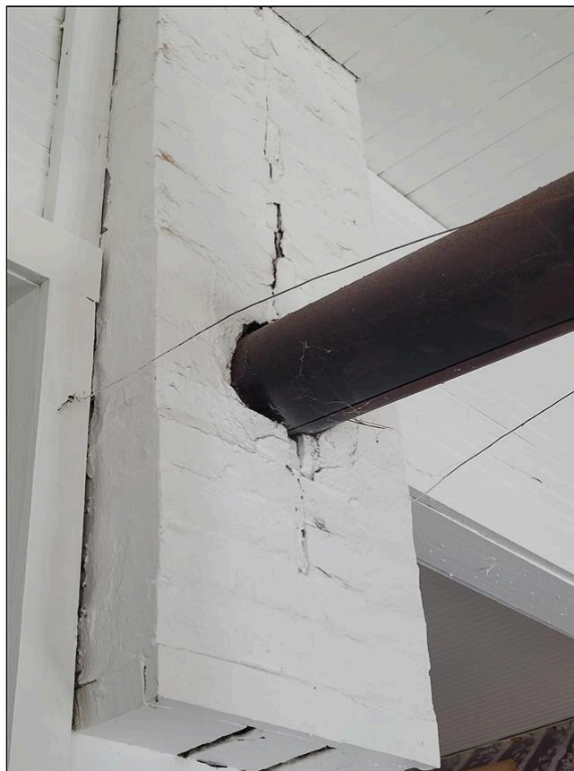
7.3 Item 2(Picture) Possible settling of bricks
