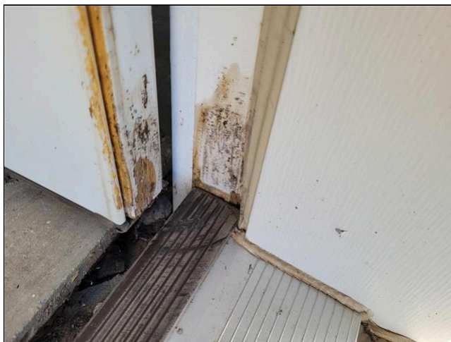
2.1 Item 6(Picture) Water intrusion-South door
