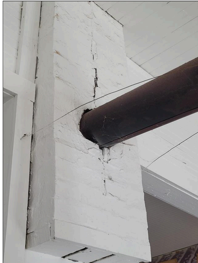
7.3 Item 2(Picture) Possible settling of bricks
