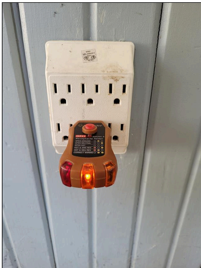
6.3 Item 1(Picture) Electrical outlets-open grounds
