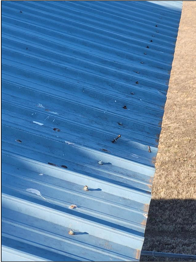
1.0 Item 2(Picture) Secure loose screws
