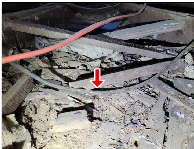
6.3 Item 2(Picture) Aged fabric wiring
