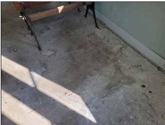
3.2 Item 1(Picture) Previous water staining
