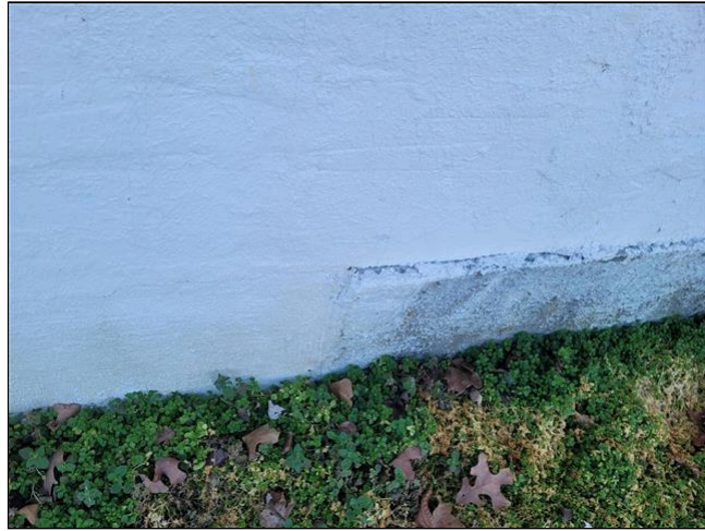
4.0 Item 4(Picture) Cracks
