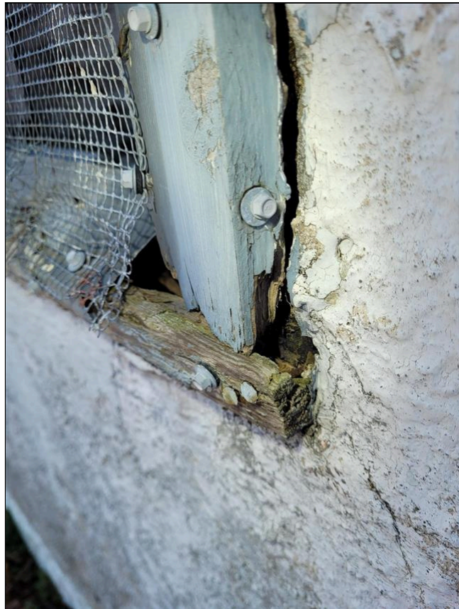
2.2 Item 4(Picture) Water intrusion likely
