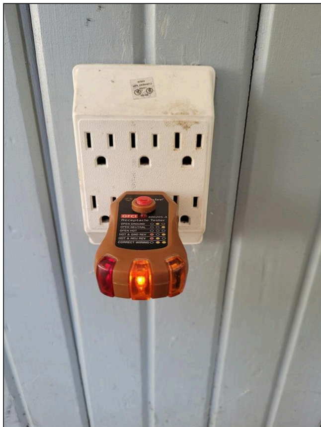
6.3 Item 1(Picture) Electrical outlets-open grounds
