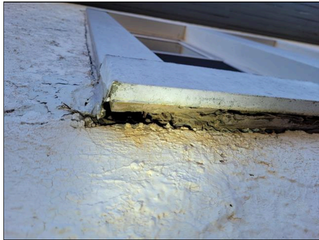
2.2 Item 2(Picture) Rotten window framing
