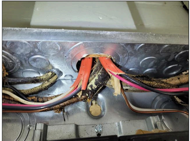
6.1 Item 3(Picture) Bushing needed
