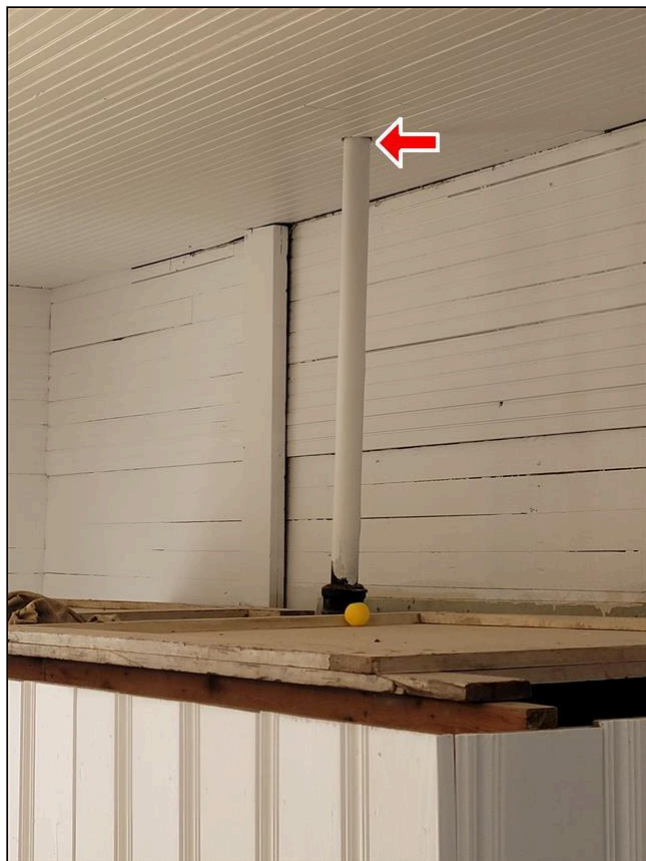
5.0 Item 1(Picture) DWV pipe-not exiting roof area
