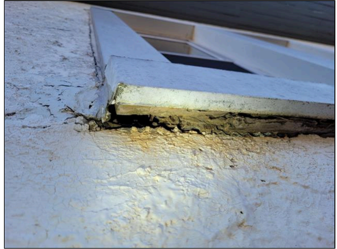
2.2 Item 2(Picture) Rotten window framing
