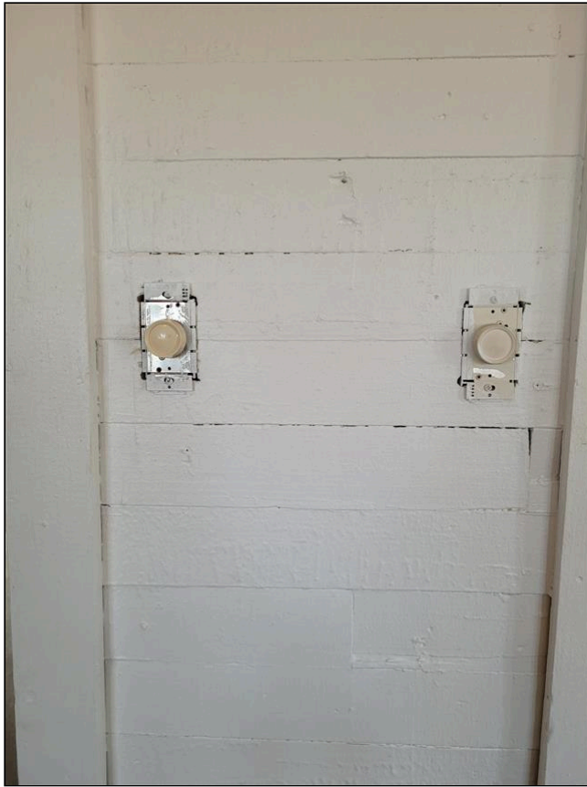
6.2 Item 1(Picture) Dimmer switches-overheating/no switch covers
