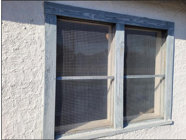
2.2 Item 5(Picture) Aged windows and trim
