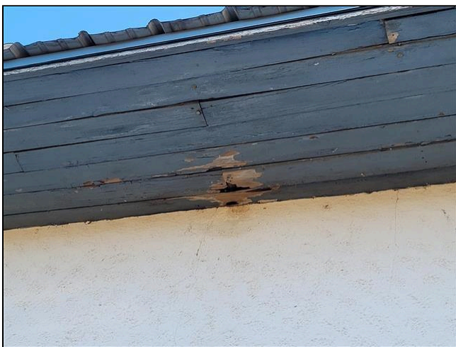
2.4 Item 5(Picture) Damaged soffit material
