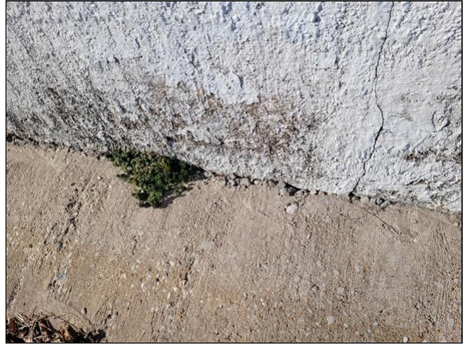
2.5 Item 2(Picture) Improper grading method
