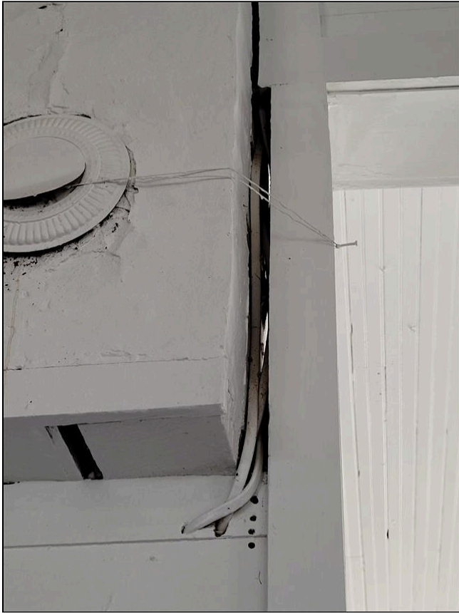
6.2 Item 3(Picture) Exposed wiring-conduit needed
