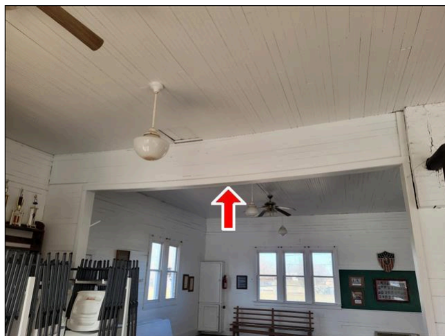
4.3 Item 4(Picture) Sagging
