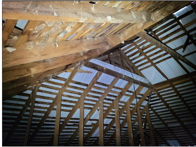
4.4 Item 4(Picture) Missing purlins
