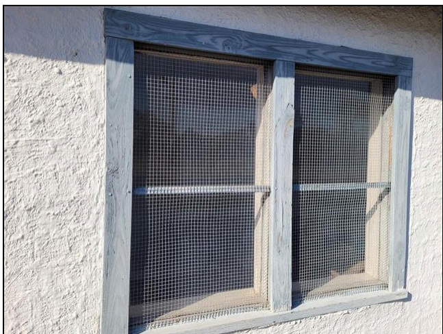
2.2 Item 5(Picture) Aged windows and trim
