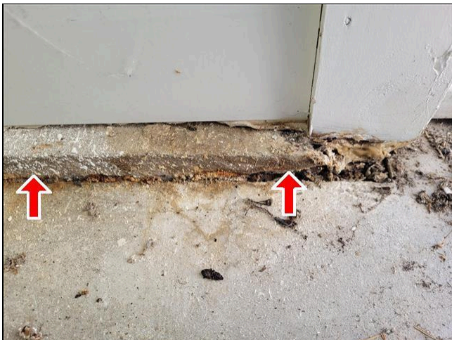
4.0 Item 1(Picture) Wood-no visible concrete footing
