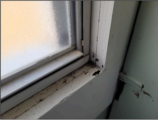
3.4 Item 1(Picture) Damaged window trim-bathroom
