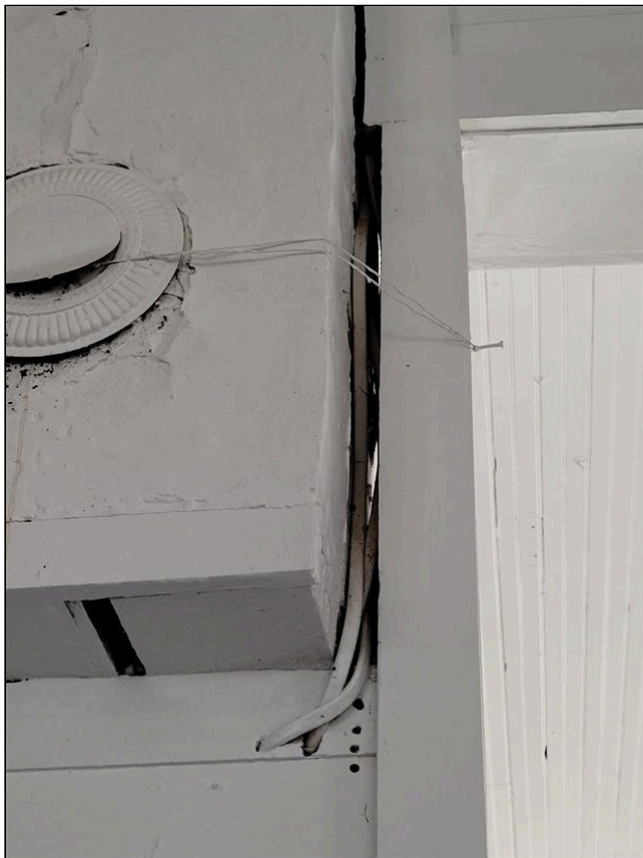
6.2 Item 3(Picture) Exposed wiring-conduit needed
