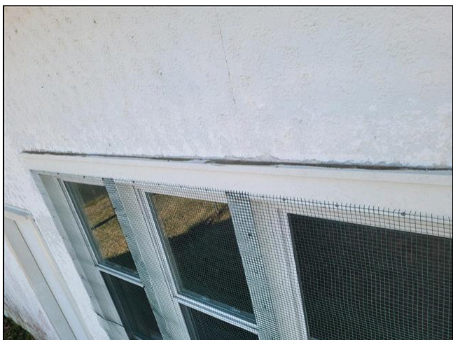
2.2 Item 7(Picture) No Z flashing-windows
