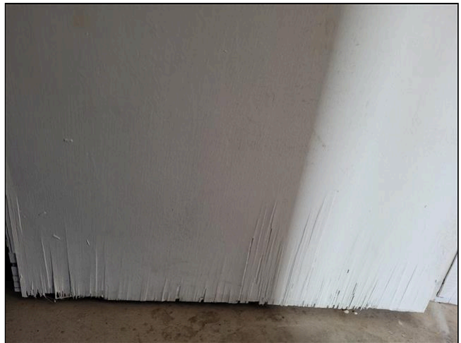
3.5 Item 4(Picture) Women's bathroom door-damaged
