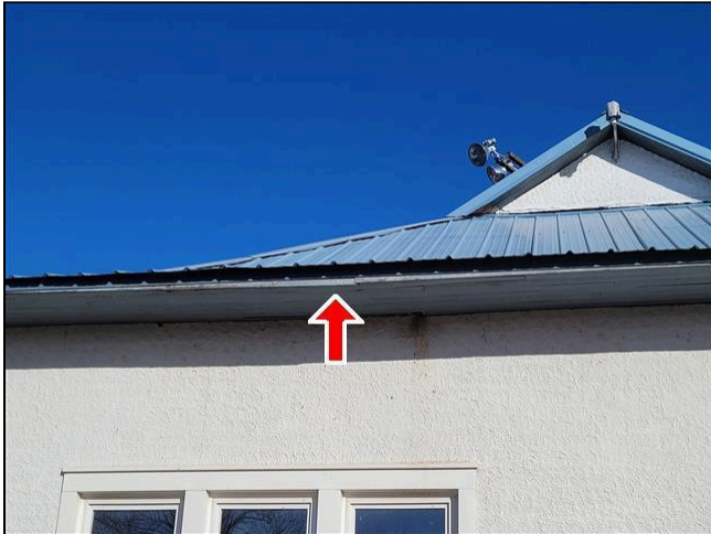
2.4 Item 3(Picture) Dropping fascia
