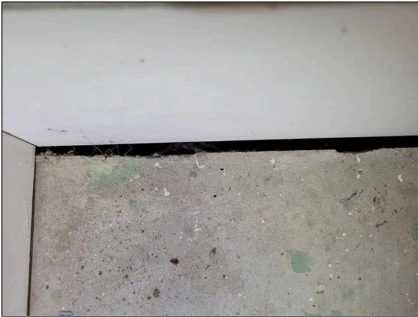
3.2 Item 3(Picture) Floor-gap in concrete
