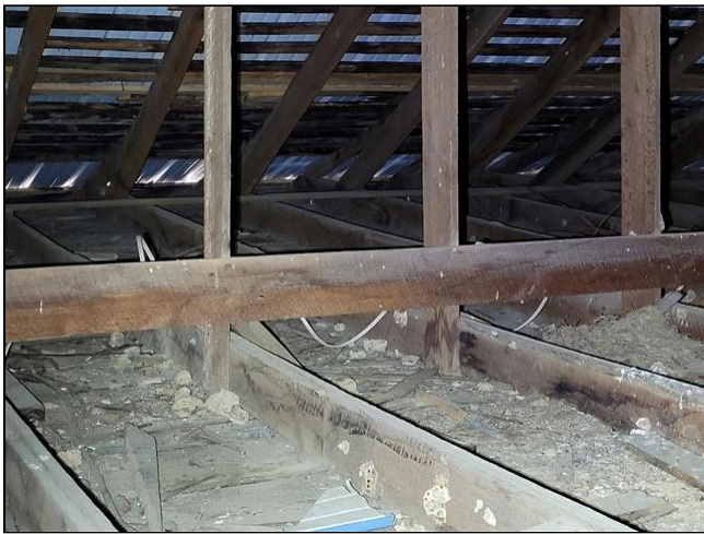
4.4 Item 5(Picture) Improper framing method
