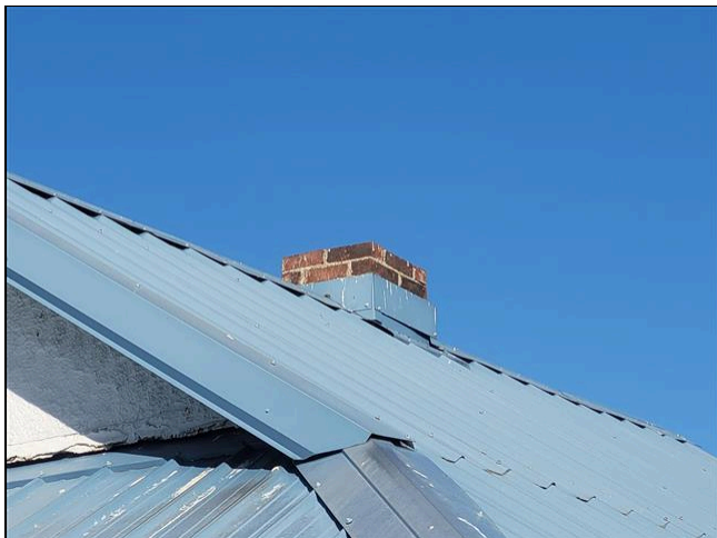
7.4 Item 1(Picture) No visible chimney cap
