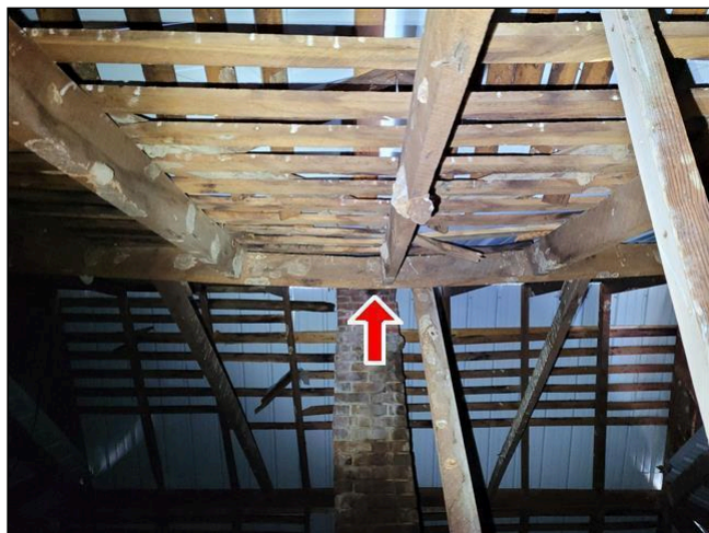
4.4 Item 1(Picture) Sagging framing area/incorrect anchoring method
