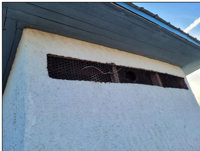
8.1 Item 1(Picture) Damaged attic vent material
