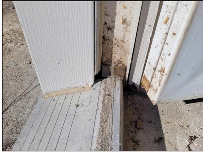
2.1 Item 2(Picture) Rotten jamb-Southeast side
