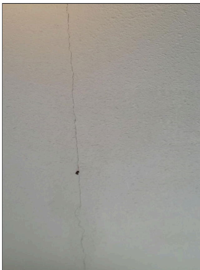
3.0 Item 4(Picture) School room ceiling-settling crack
