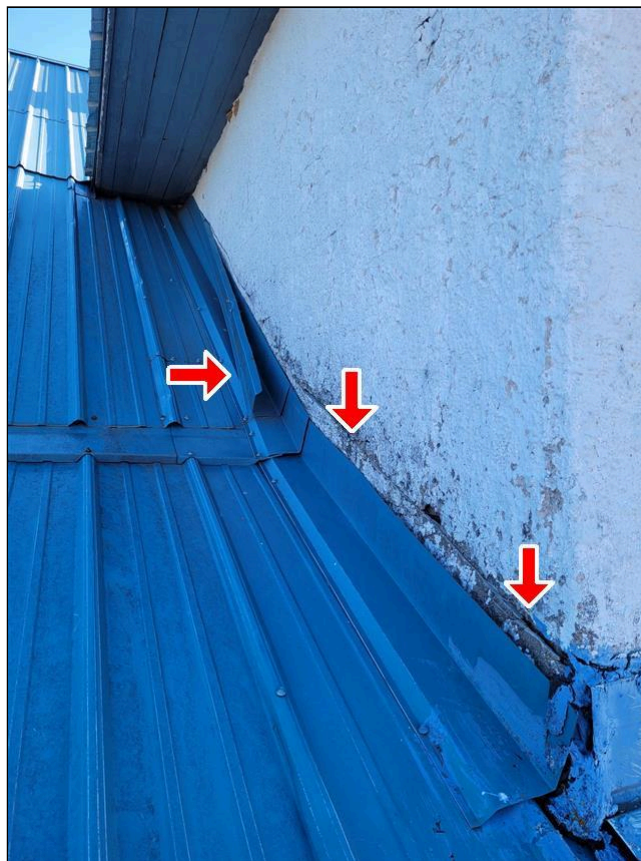
1.1 Item 8(Picture) Loose/missing flashing
