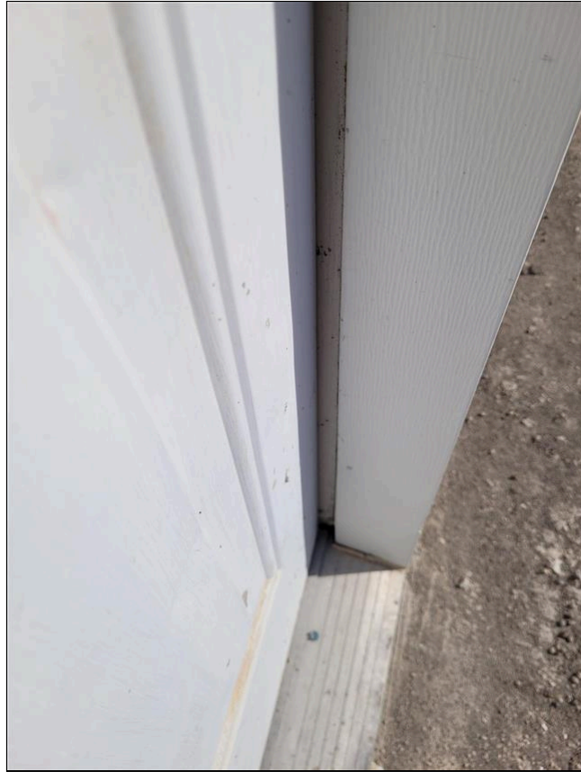
2.1 Item 8(Picture) Unsealed door-Southeast door
