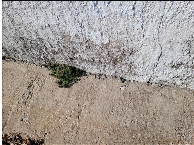
2.5 Item 2(Picture) Improper grading method
