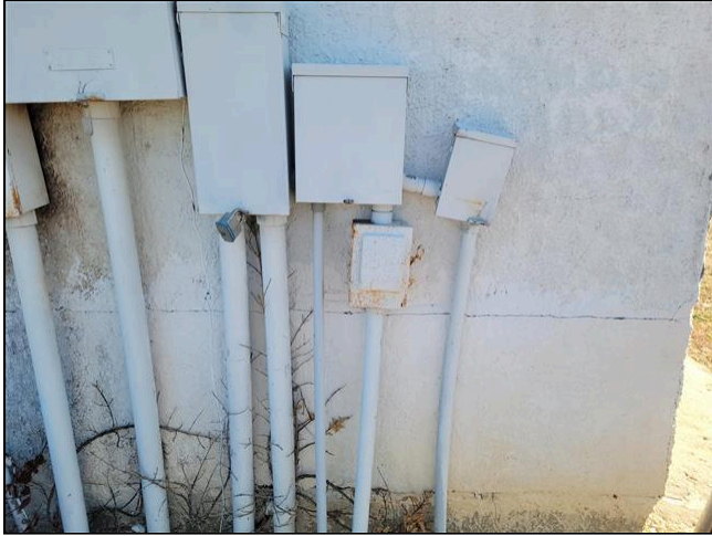
2.0 Item 1(Picture) Cracked exterior
