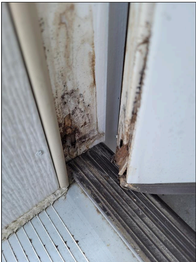
2.1 Item 5(Picture) Rotten jamb, rotten door-North door
