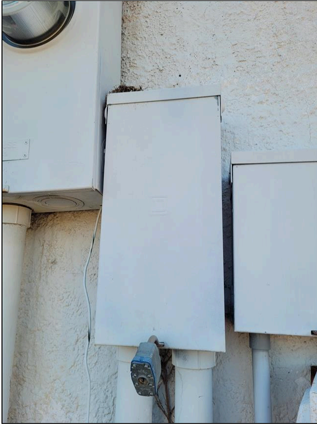
6.1 Item 1(Picture) Locked-not inspected
