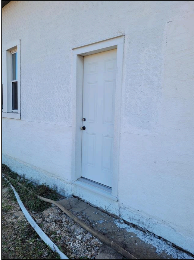
2.3 Item 1(Picture) Step and handrail needed-West side
