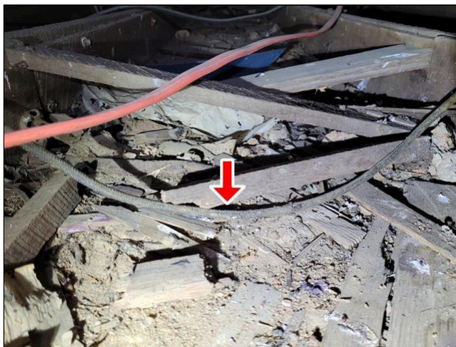
6.3 Item 2(Picture) Aged fabric wiring
