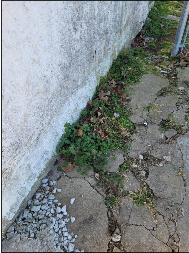
2.5 Item 1(Picture) Improper grading method
