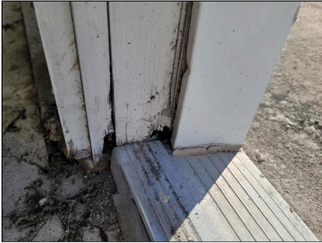
2.1 Item 1(Picture) Rotten jamb-Southeast side
