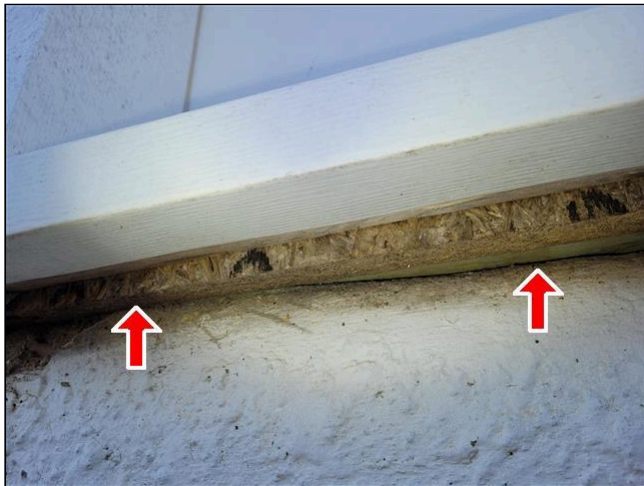
2.1 Item 9(Picture) No visible flashing
