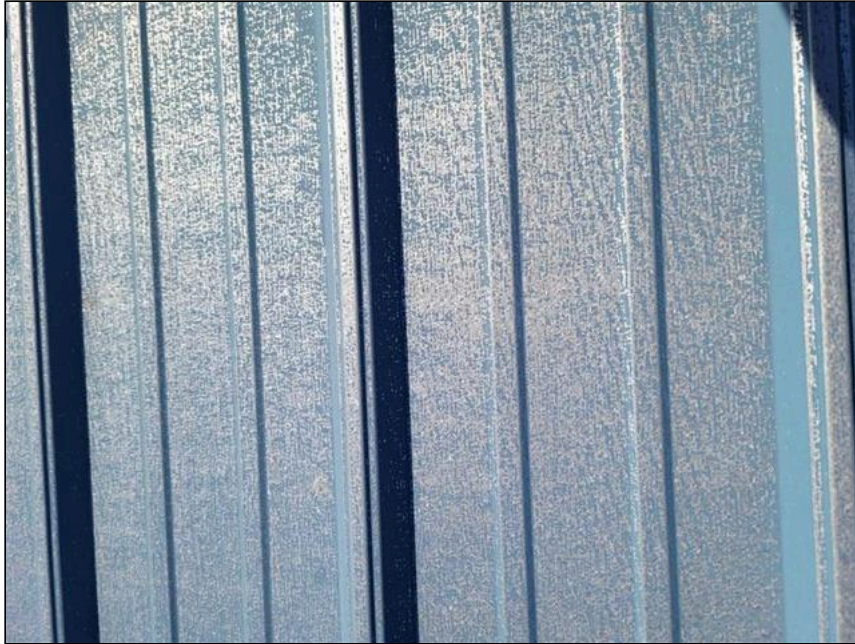
1.0 Item 1(Picture) Paint-coming off
