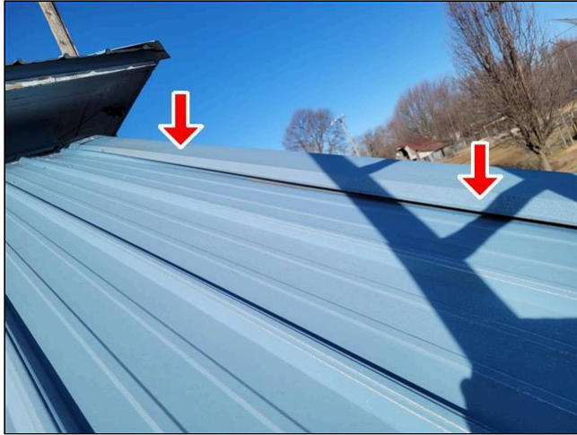
1.0 Item 4(Picture) Missing screws
