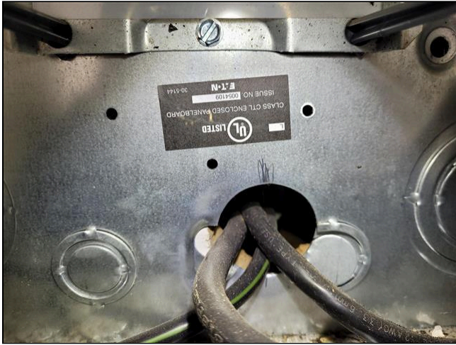
6.1 Item 4(Picture) Bushing needed
