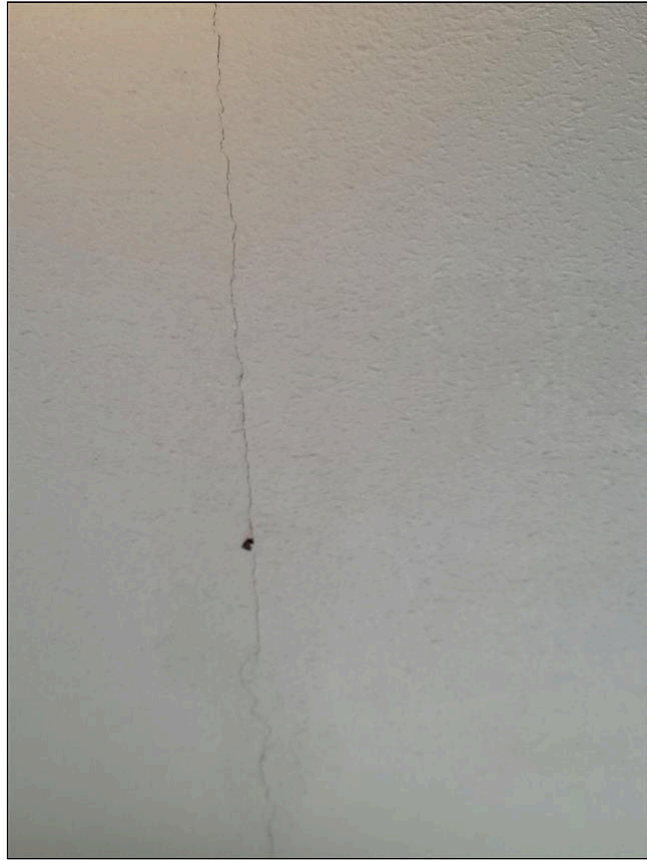
3.0 Item 4(Picture) School room ceiling-settling crack
