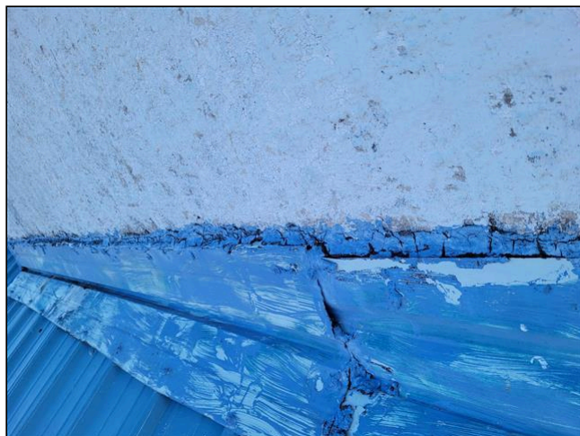
1.1 Item 7(Picture) Cracked sealant
