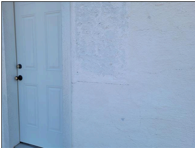
2.0 Item 3(Picture) Cracked exterior
