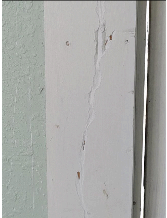
3.4 Item 2(Picture) East school room trim-possible would destroying insect damage
