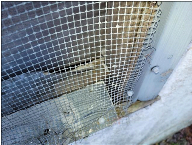
2.2 Item 3(Picture) Missing pane-North side
