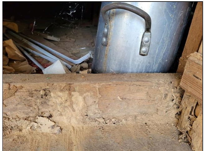
3.7 Item 4(Picture) Wood destroying insect activity
