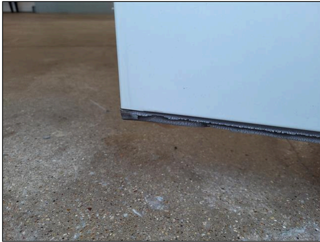
2.1 Item 7(Picture) Replace all damaged threshold seals
