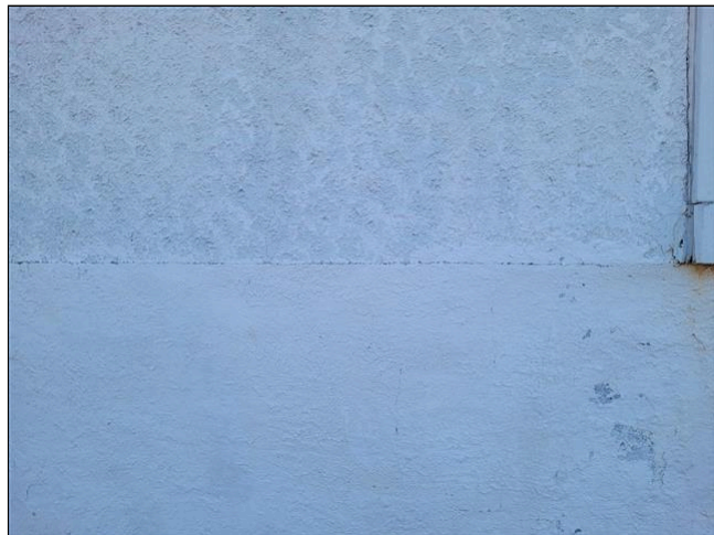
2.0 Item 4(Picture) Cracked exterior
