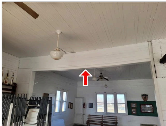
4.3 Item 4(Picture) Sagging
