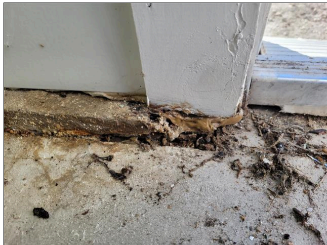
4.0 Item 2(Picture) Wood destroying insect activity
