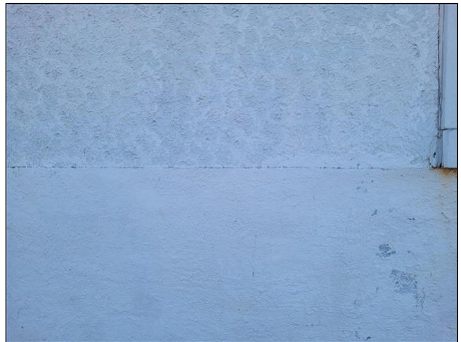
2.0 Item 4(Picture) Cracked exterior
