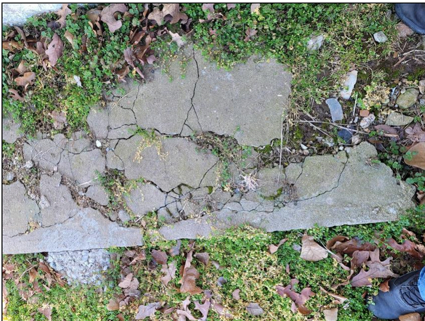
2.5 Item 5(Picture) Damaged concrete
