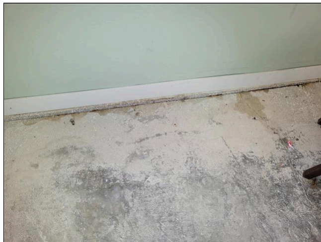
3.2 Item 2(Picture) Previous water staining
