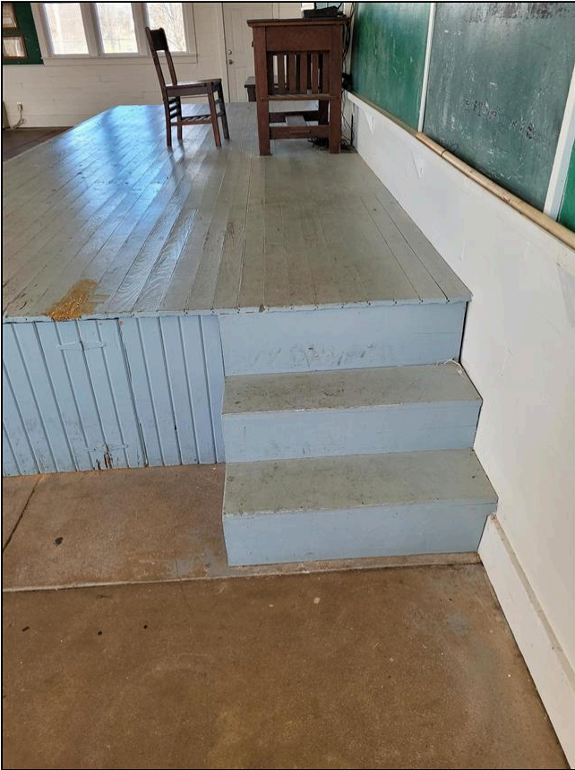
3.3 Item 1(Picture) Handrail-needed for the stage
