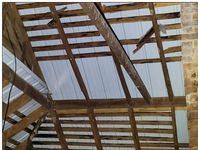
4.4 Item 2(Picture) Missing purlins
