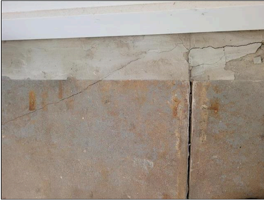
3.2 Item 7(Picture) Floor-settling cracks
