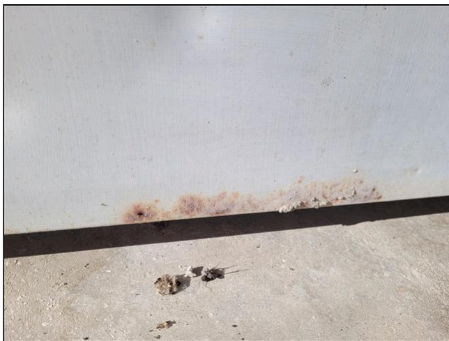
2.1 Item 3(Picture) Rust holes-Southeast side
