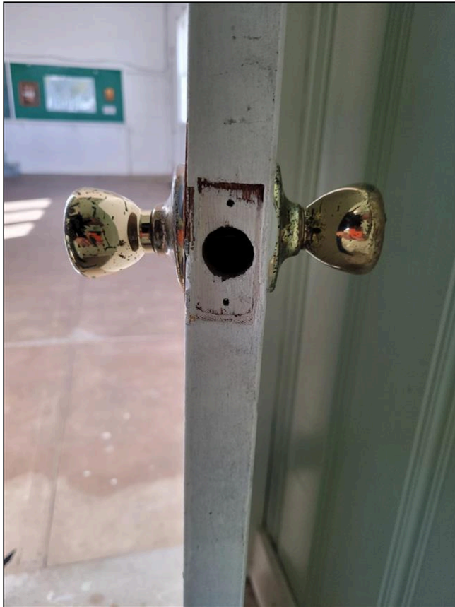
3.5 Item 1(Picture) Men's bathroom door-missing latch
