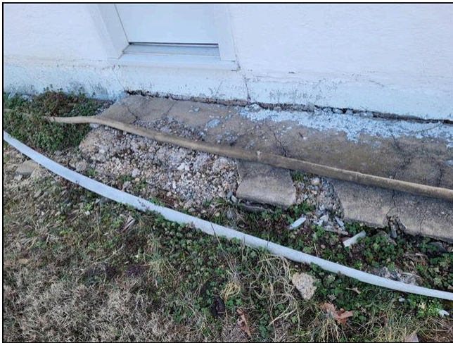
2.5 Item 4(Picture) Damaged concrete
