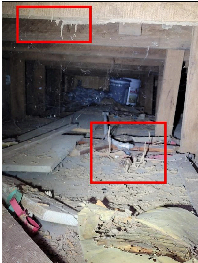
3.7 Item 2(Picture) Wood destroying insect activity
