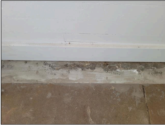
4.0 Item 6(Picture) Exterior wall-slab area not continuous
